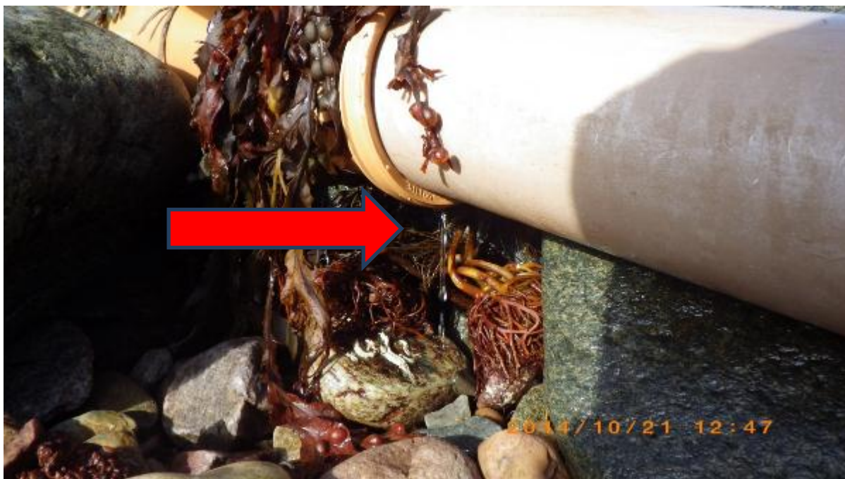
Figure 13. Associated with waypoints 58 and 59. Location of unplanned freshwater sample SFFW8 from leak in pipe.
