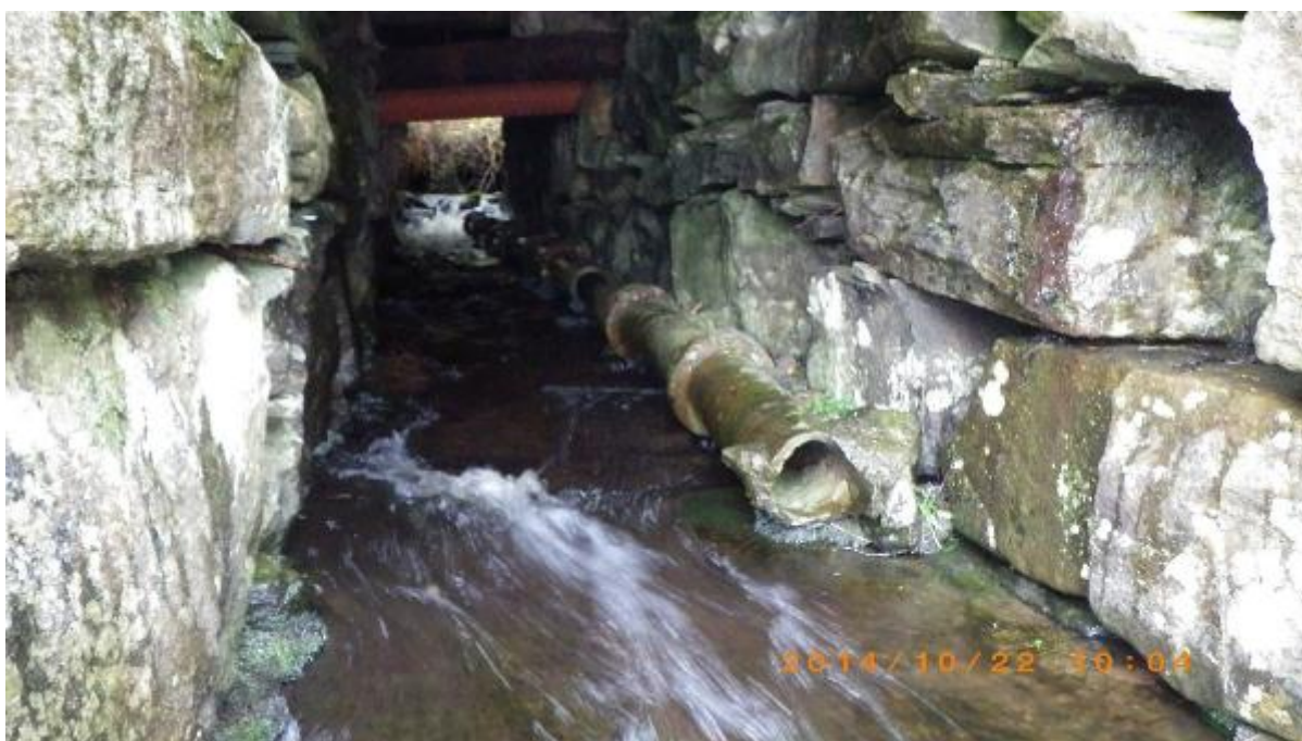
Figure 14. Associated with waypoints 67 and 68. Location of unplanned freshwater sample SFFW11 from culvert.
