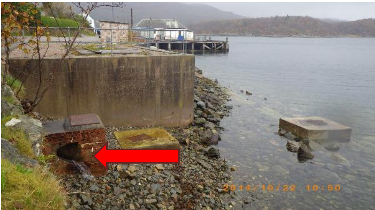
Figure 16. Associated with waypoints 81 and 82. Location of unplanned freshwater sample SFFW15 from pipe.
