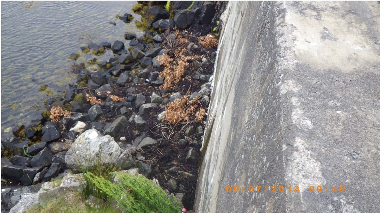
Figure 6. Pipe from under road, historical evidence of flow. Waypoint 17.
