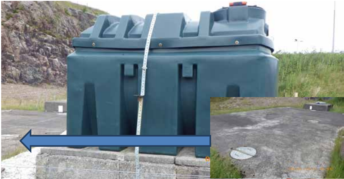
Figure 5. Container and manhole covered area at location marked on map as Kinlochbervie septic tank. Waypoint 25.
