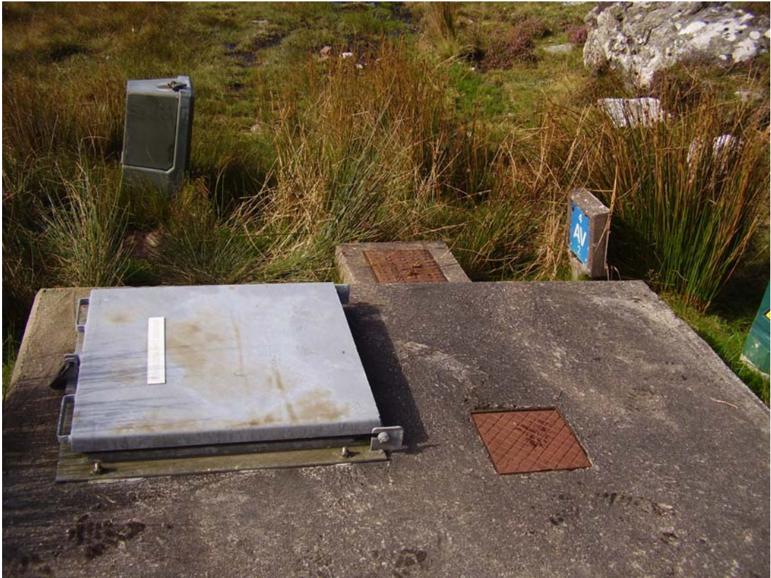
Figure 30. Innis Place septic tank
