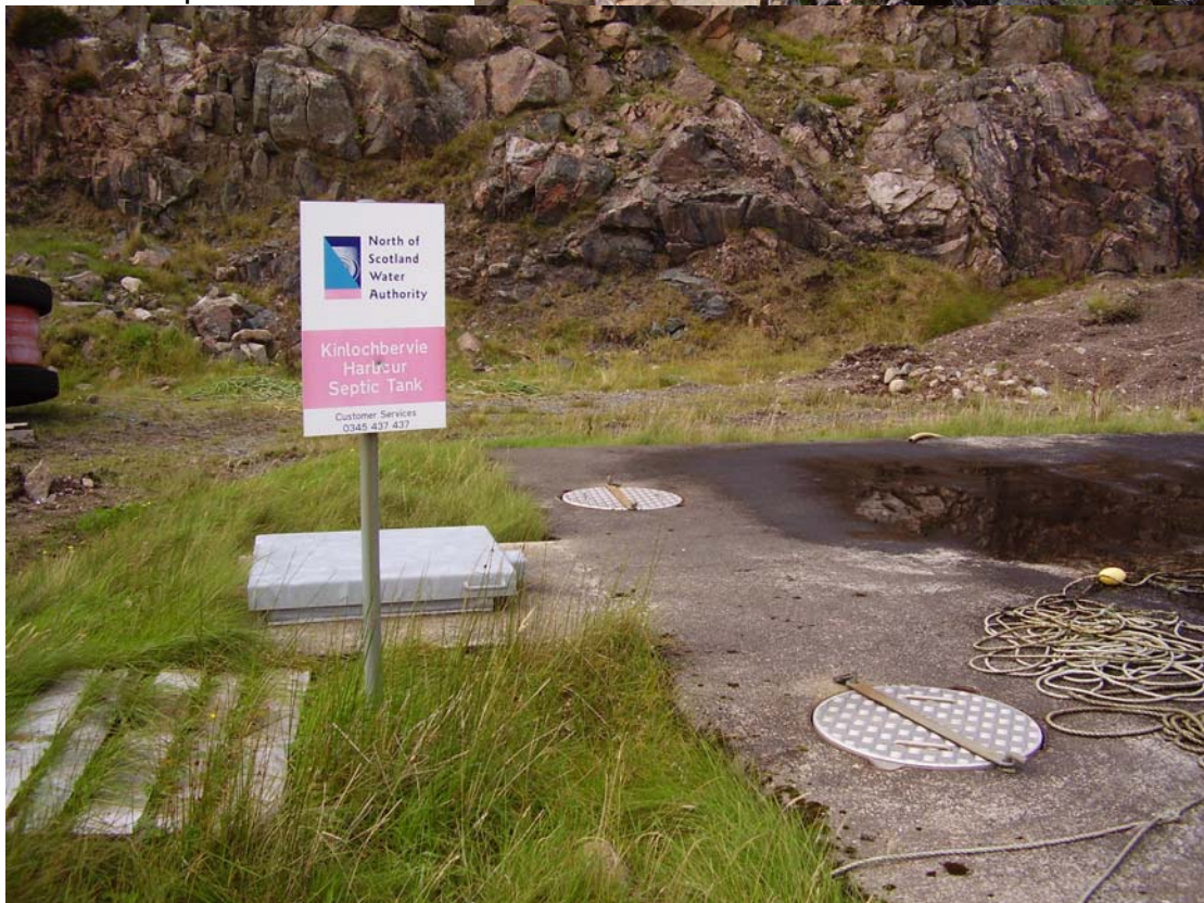
Figure 23. Kinlochbervie Harbour Septic Tank.
