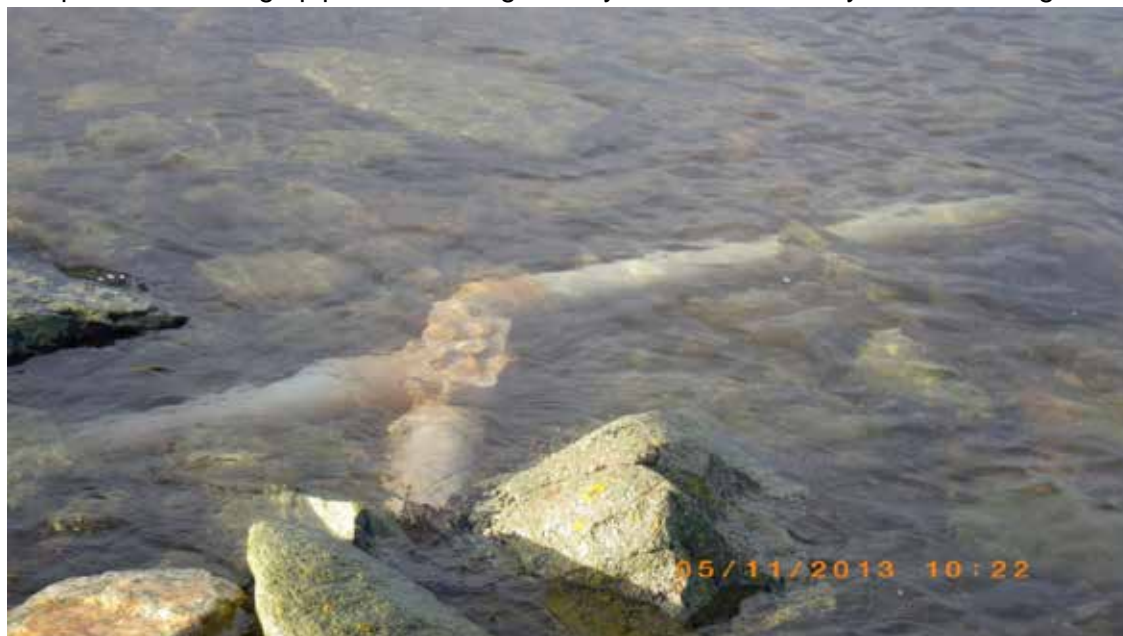
Fig 4. Joint discharge pipe running into water below site of Caravan Park (waypoint 4)
