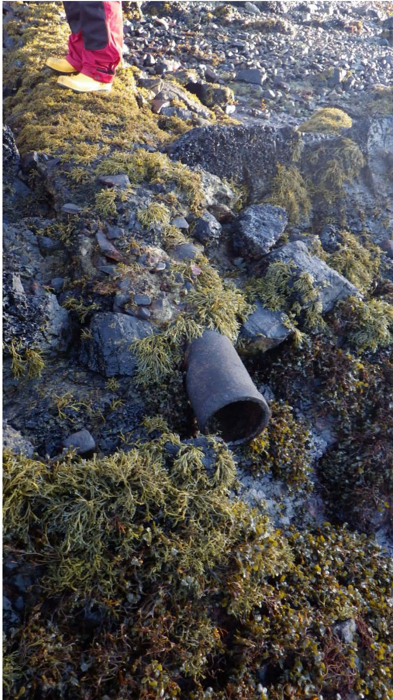
Figure 26: Cast iron pipe on shore with no evident outflow (Waypoint 38)
