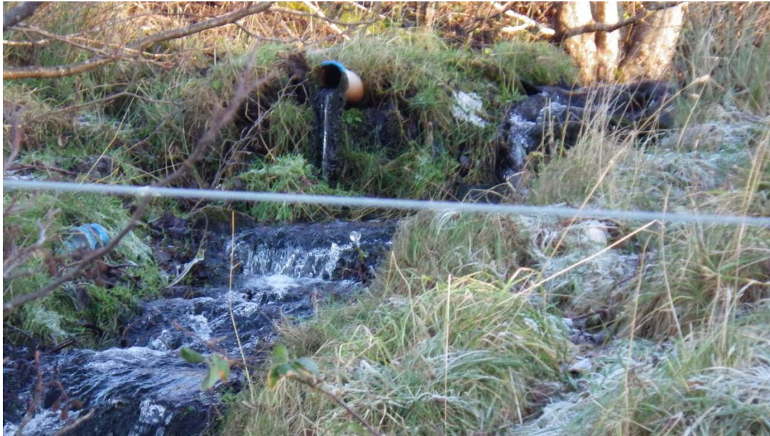
Figure 30: Plastic outfall pipe visible behind fence discharging into stream. (Waypoint 40)
