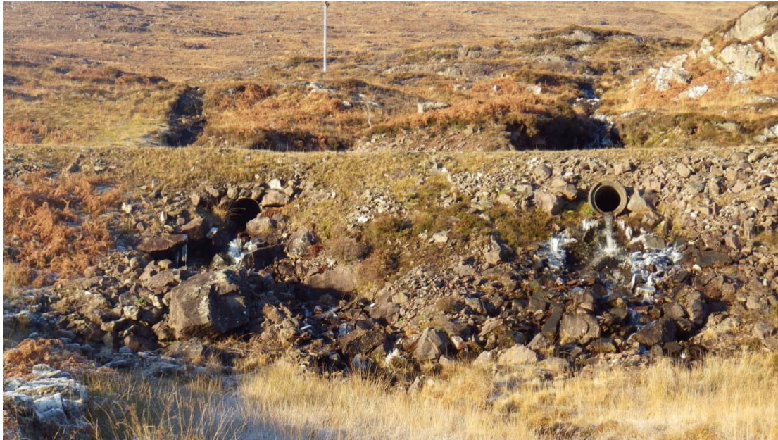
Figure 22: Two concrete pipes running under road and discharging on to shore (Waypoint 31)
