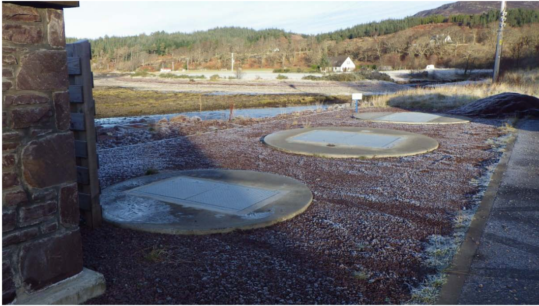
Figure 10: Kishorn Achintraid CSO (Waypoint 11)
