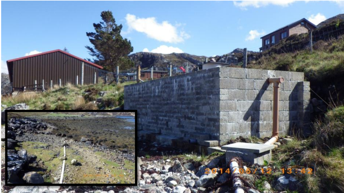
Fig 14. Septic tank at Ardmore Adventure School Skerricha shore survey waypoint 21. Insert picture associated with Waypoint 23 and unplanned seawater sample LLSW1. Skerricha shore survey.
