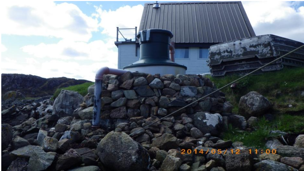
Fig 6. Septic tank with shore outfall. Waypoint 4.
