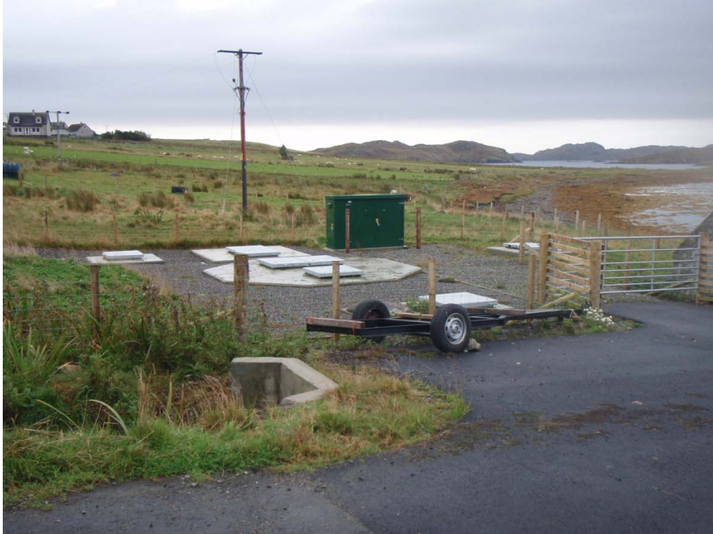
Figure 5. Newer septic tank at Crosbost
