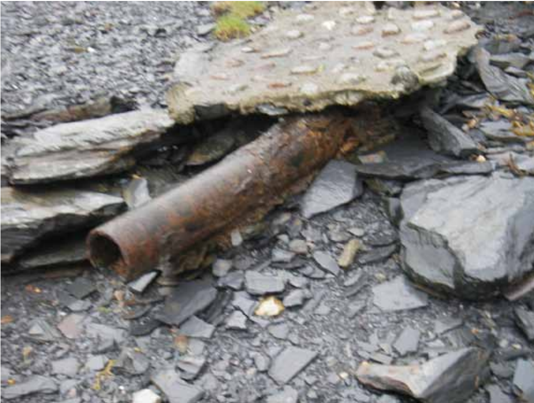
Figure 7. Possibly disused pipe by hotel
