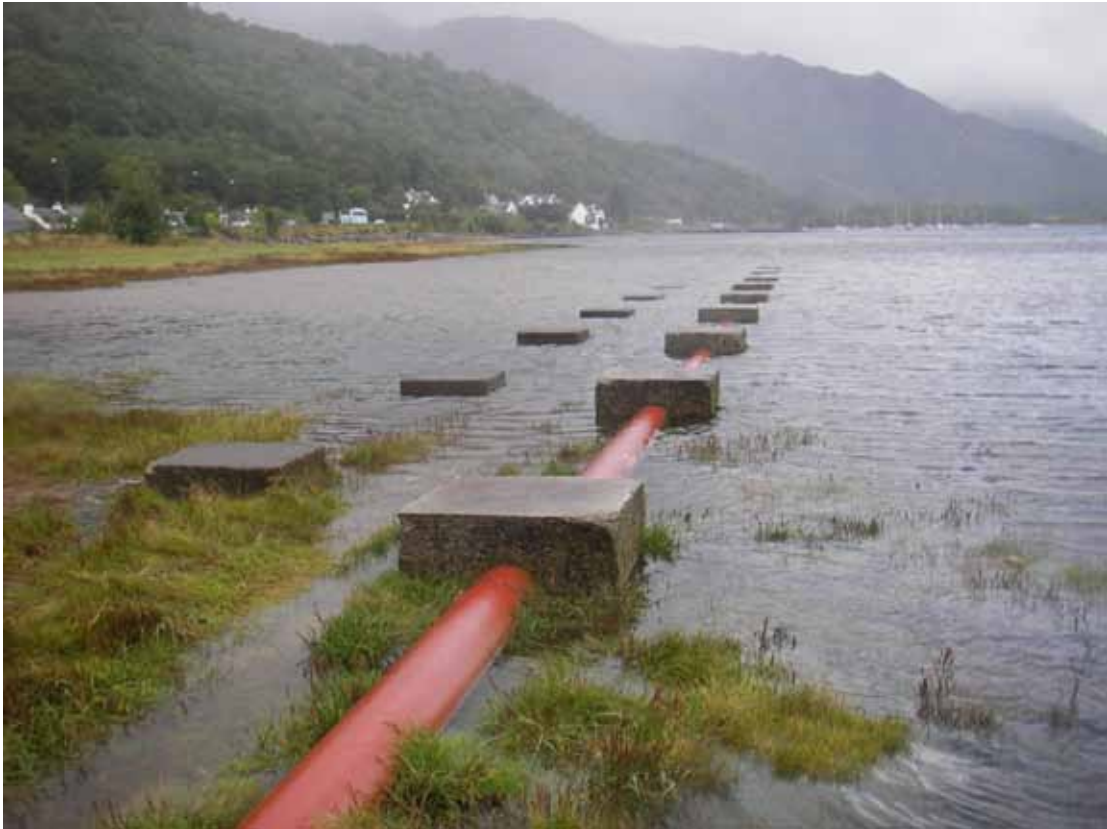
Figure 11. Pipes running out from Glencoe WWPS
