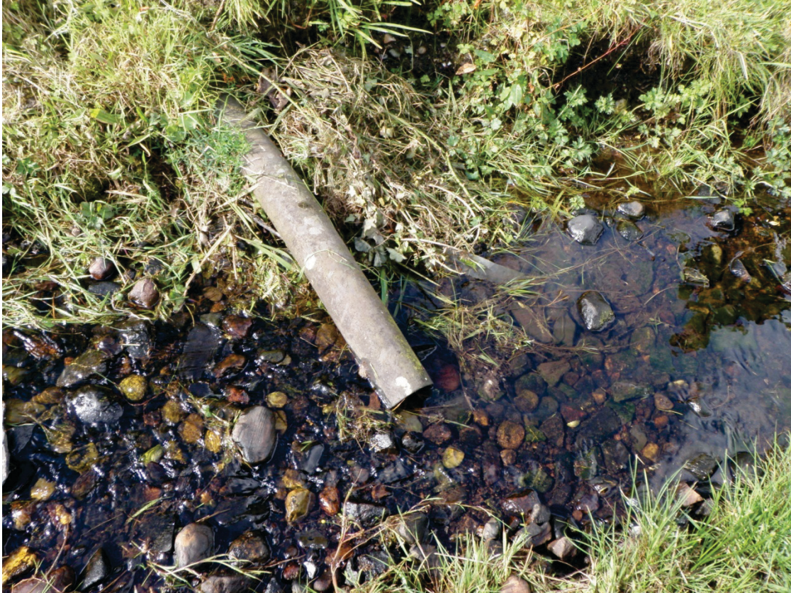
Figure 12. Outfall pipe flowing into stream previously sampled (LINNHE FW2)
