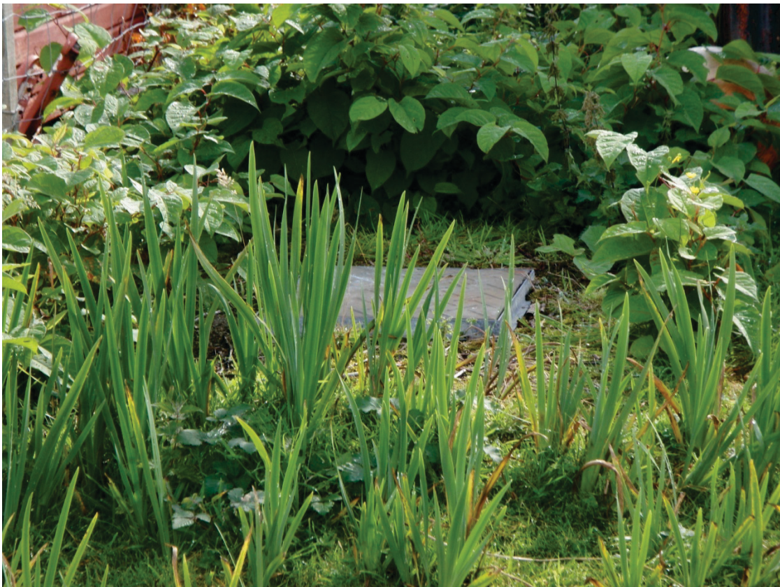
Figure 13. Septic tank, no sign of outfall pipe
