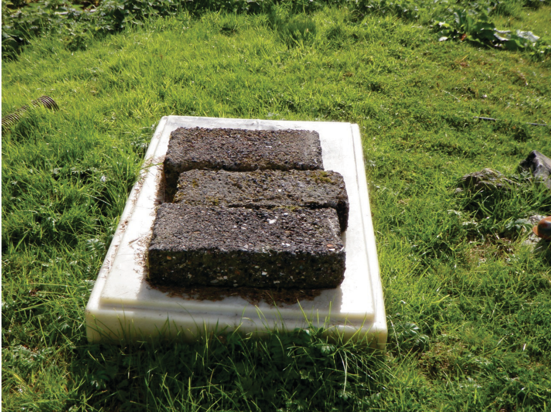
Figure 10. Septic tank, no sign of outfall pipe
