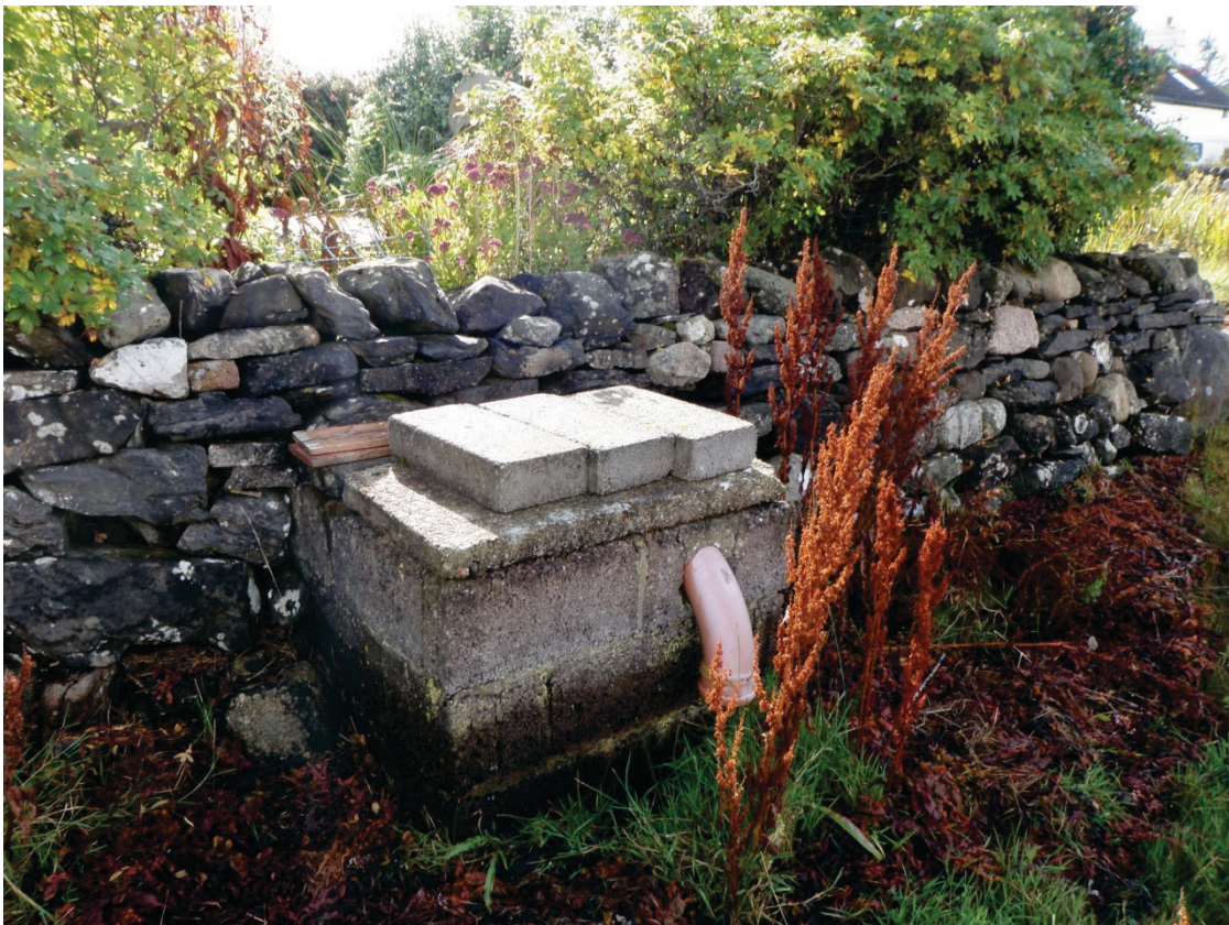
Figure 15. Septic tank and pipe, no flow
