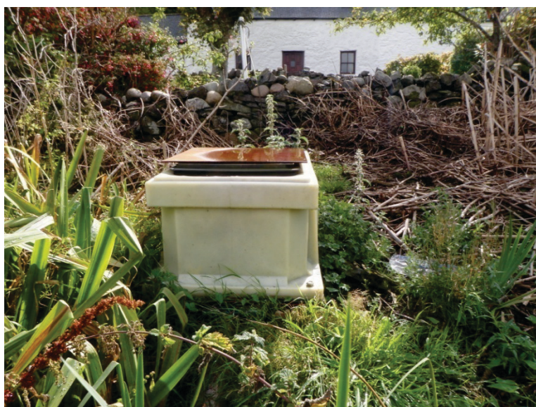
Figure 9. Septic tank, no sign of outfall pipe
