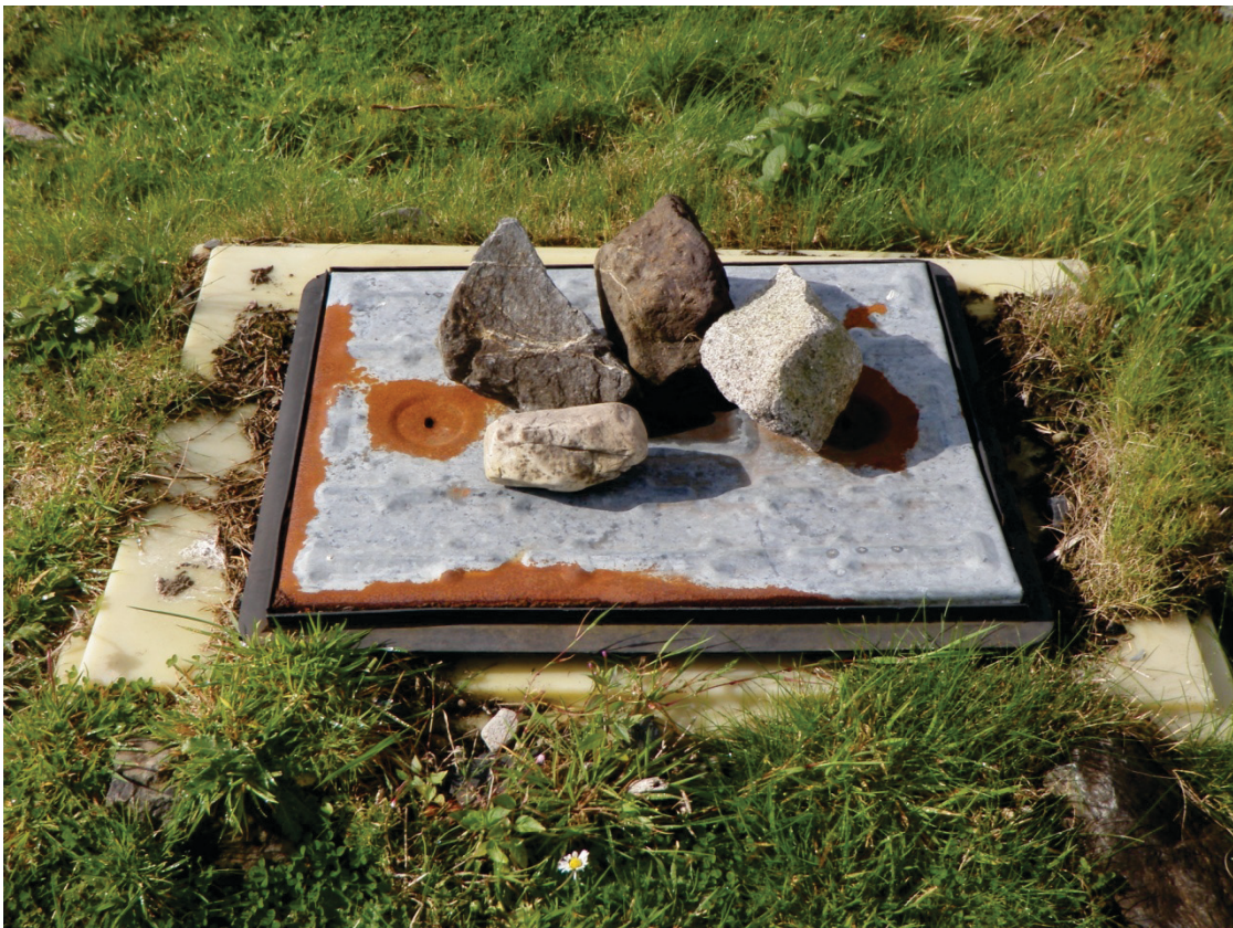
Figure 11. Septic tank, no sign of outfall pipe
