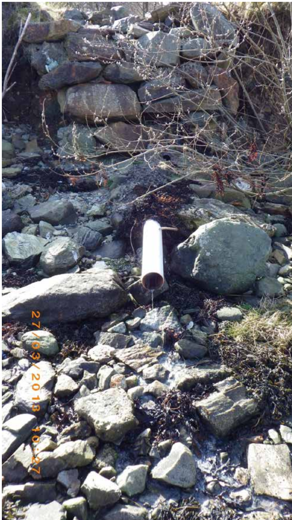
Figure 12. Waypoint 51. Plastic outflow pipe, smelling strongly of sewage. Site of sample LNCFW13.
