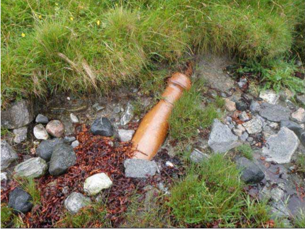
Figure 8. Ceramic septic pipe
