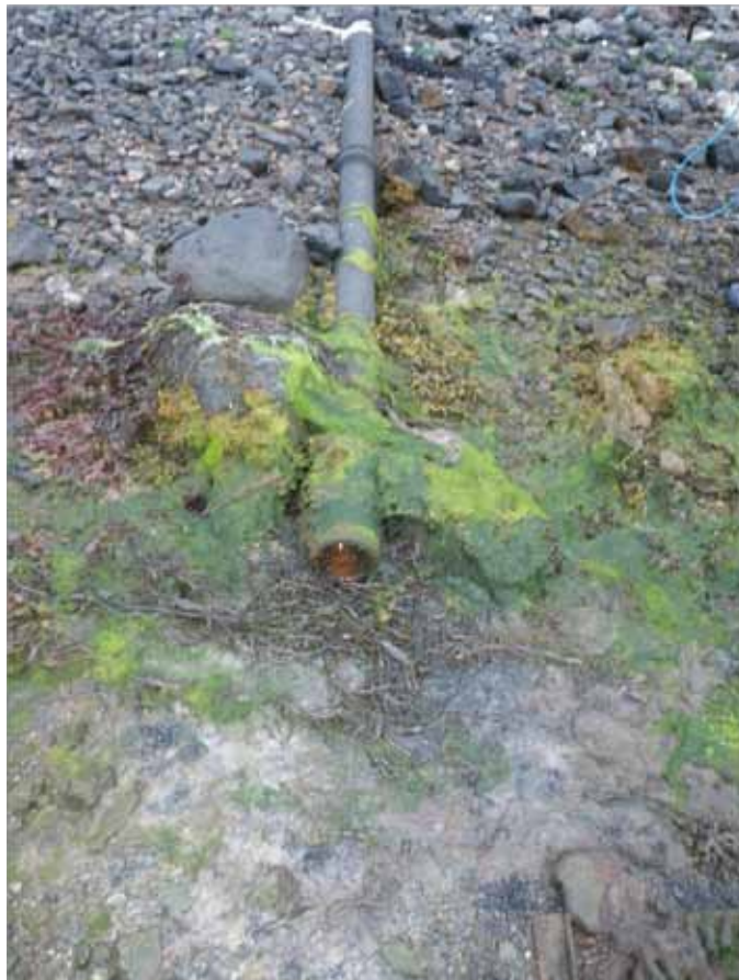
Figure 9. Septic discharge from church at Loch Miavaig
