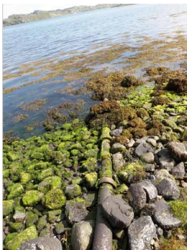
Figure 15. Cast iron discharge pipe
