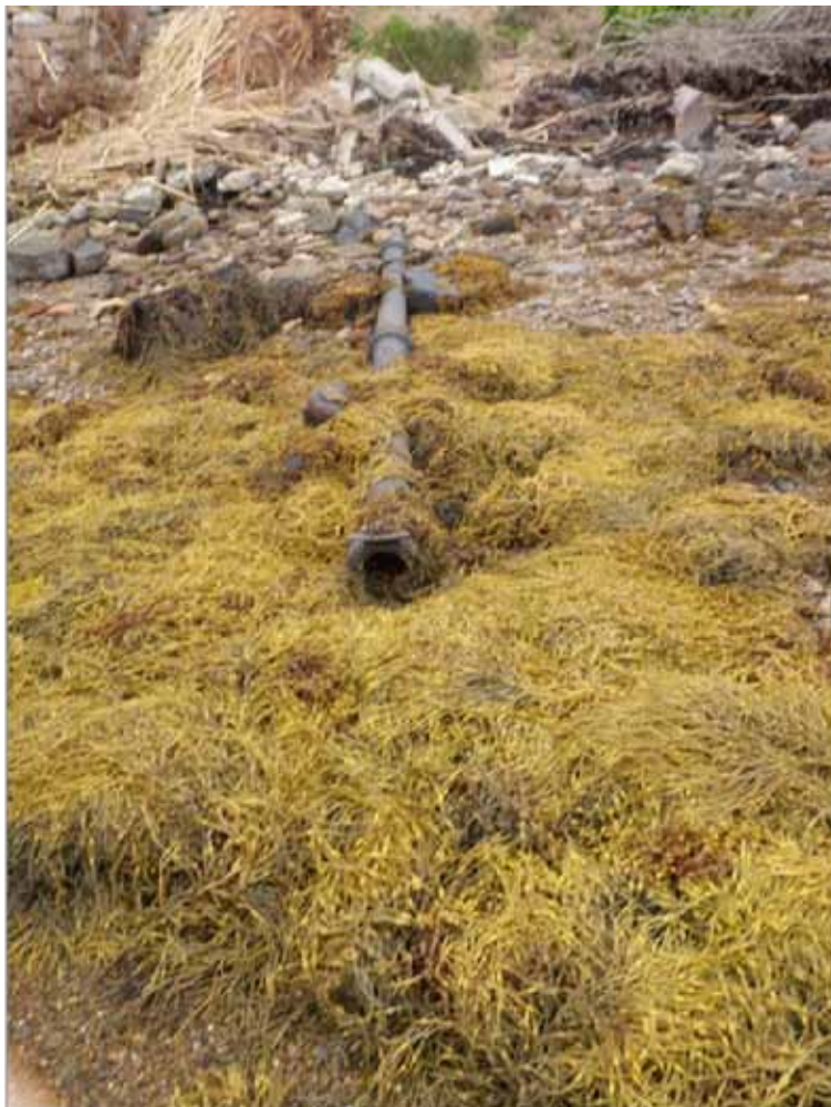
Figure 11. Iron discharge pipe below house
