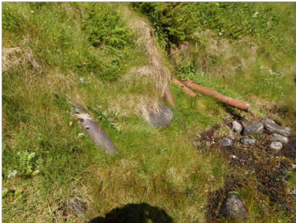
Figure 14. Four discharge pipes
