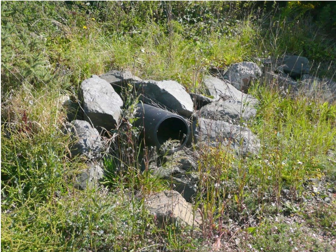
Figure 19. Black outfall pipe – dry
