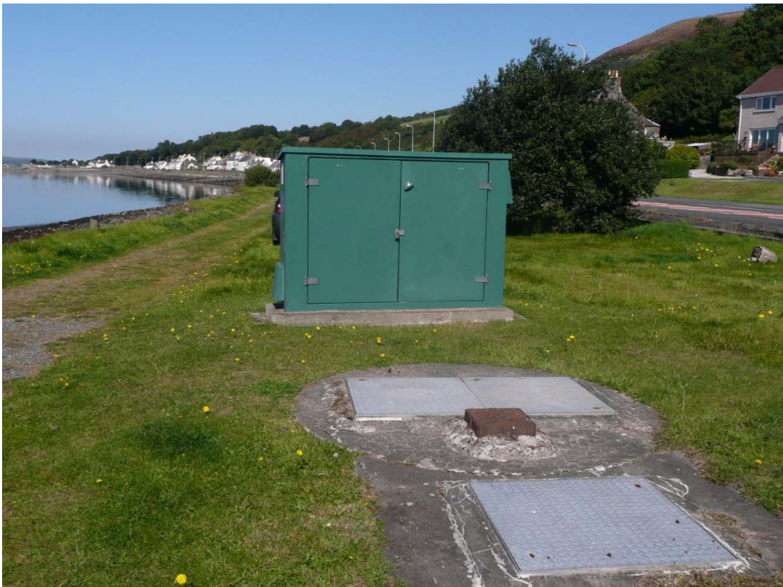
Figure 17. Septic tank outflow 3
