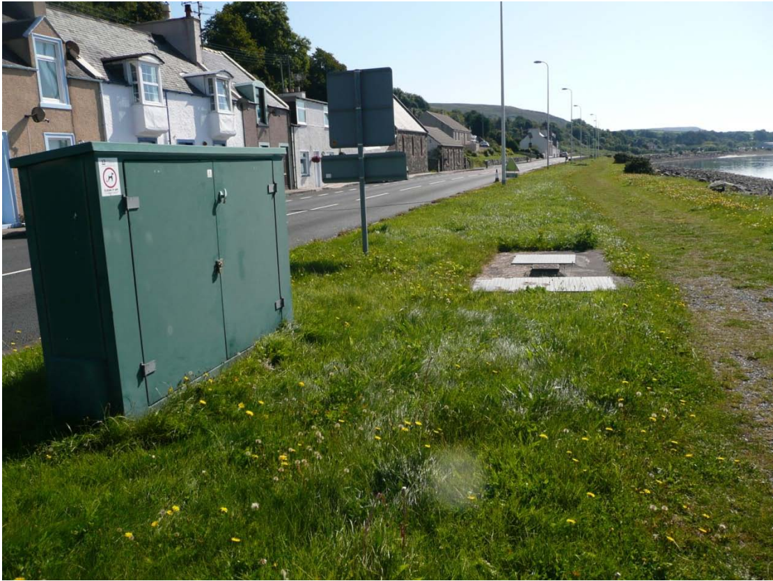
Figure 16. Septic tank outflow 2
