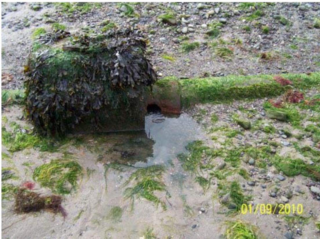
Figure 5. Sewage outfall pipe, location of water sample LR001
