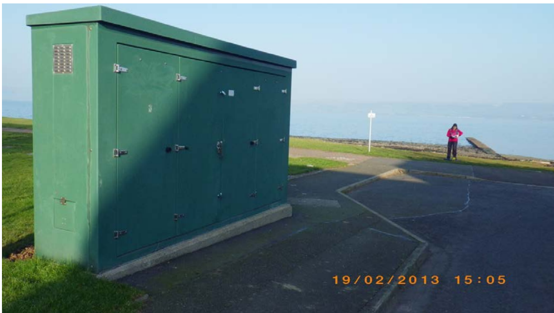
Figure 18. Pumping station with pipe running into sea. Waypoint 26.
