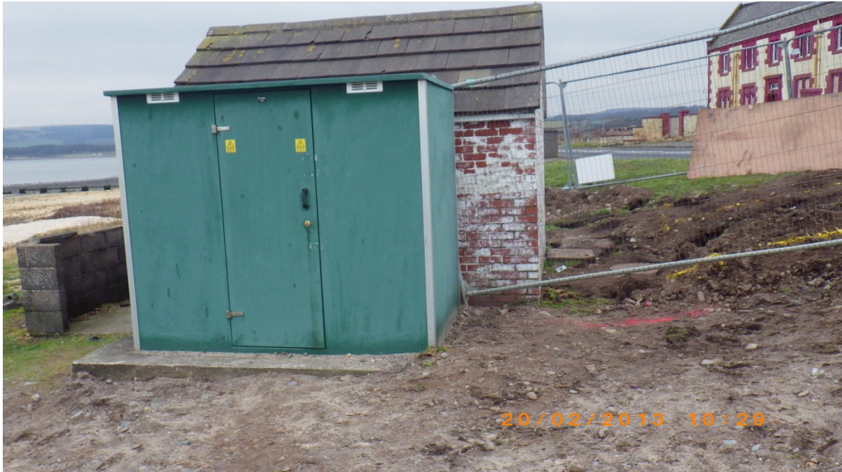
Figure 25. Pumping station on shore with manhole covers. Waypoint 37.
