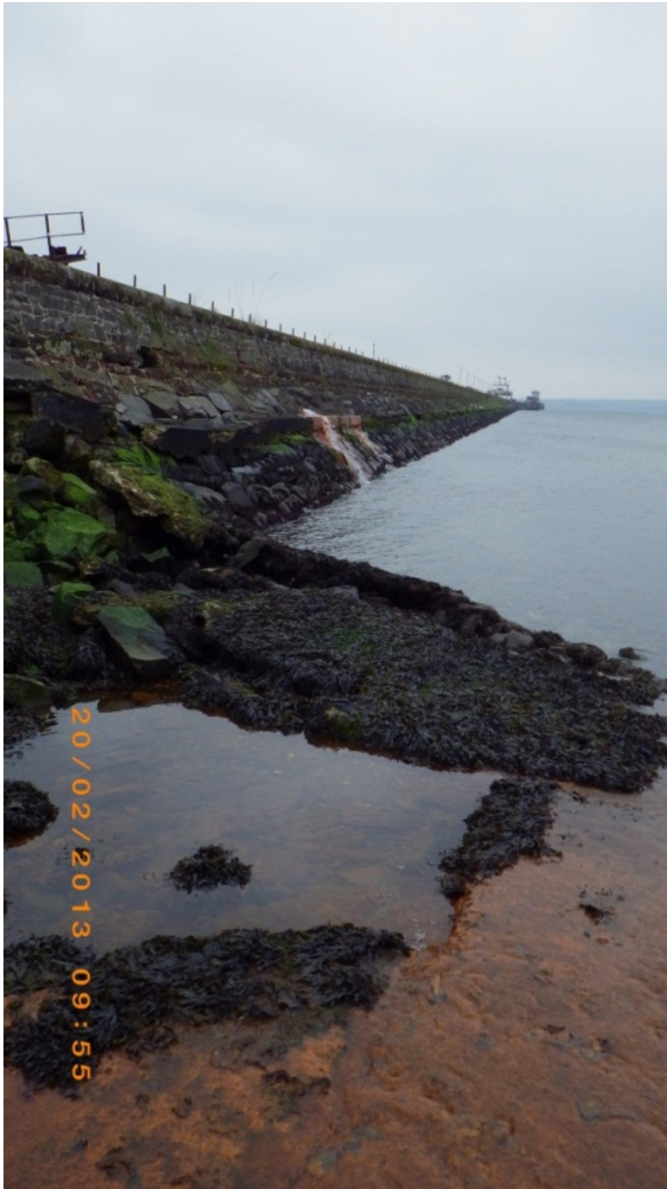
Figure 21. Outflows from under railway line. Waypoint 31.
