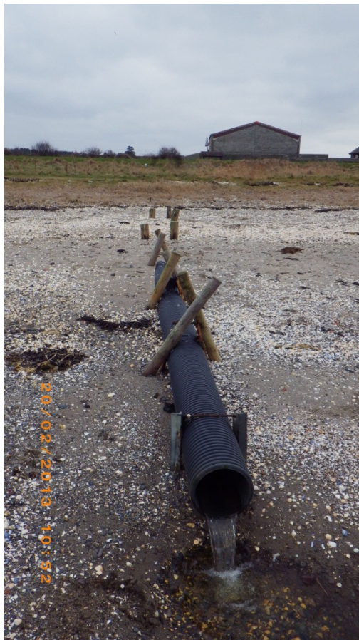
Figure 28. Plastic pipe with yellowish discharge runs onto shore. Waypoint 41.
