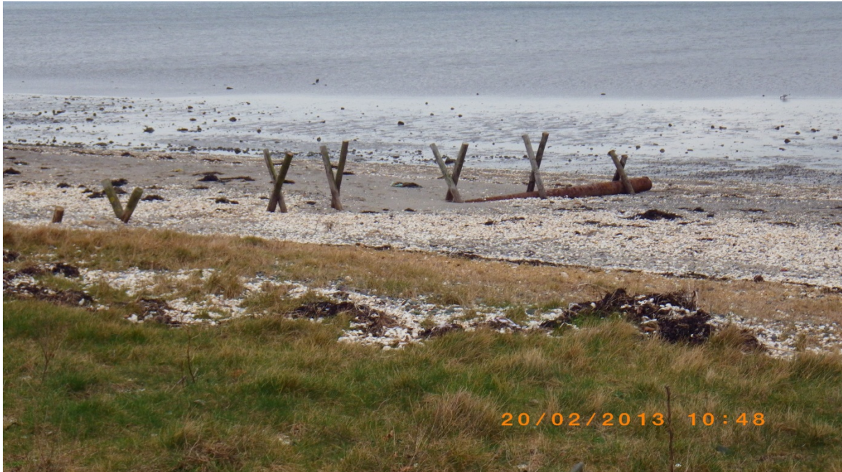
Figure 27. Metal pipe on shore with no discharge. Waypoint 40.
