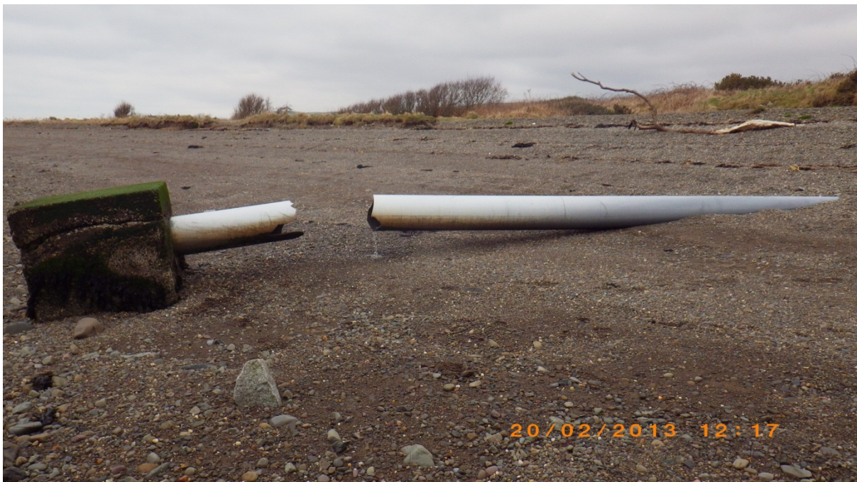
Figure 30. Broken plastic pipe runs onto shore from under the road. Waypoint 48.
