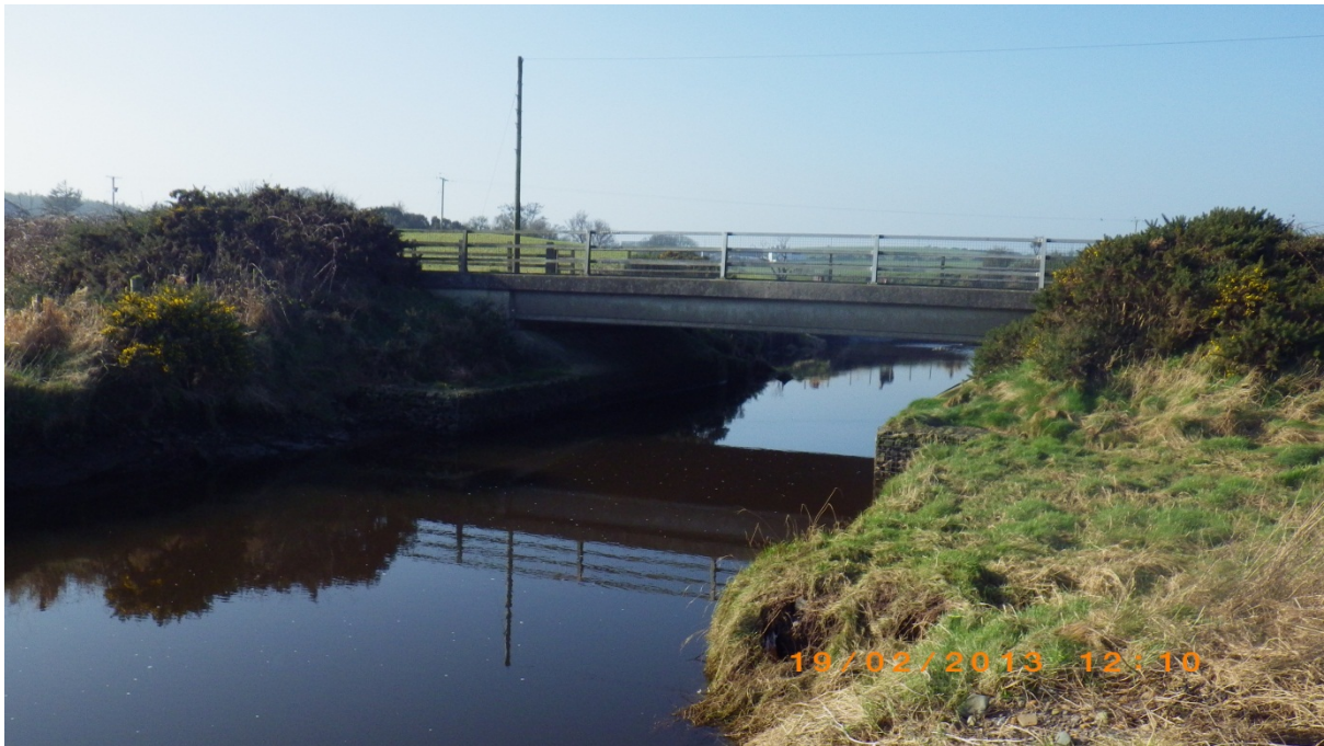
Figure 9. Sole Burn with bridge. Waypoint 14.
