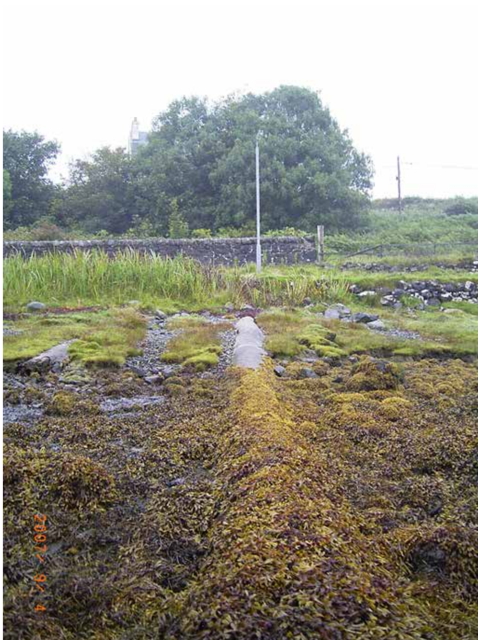
Figure 10. Private sewer pipes at Bunessan
