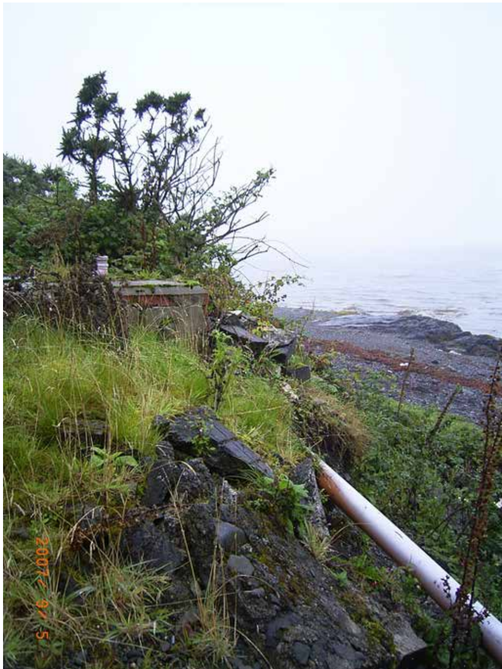
Figure 15. Septic tank with overflow to beach
