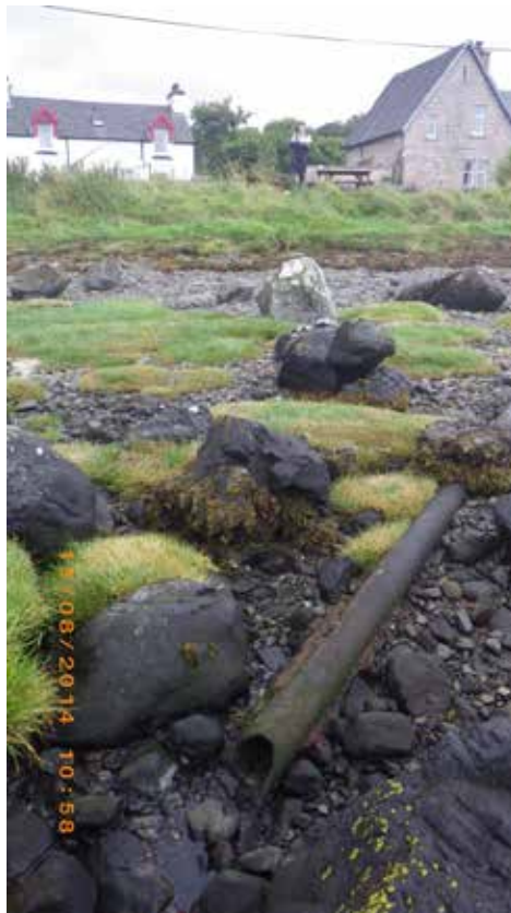
Figure 16: Discharge pipe on foreshore at Pennyghael (WP 69). Building on the right hand side of photo is Pennyghael Village Hall.
