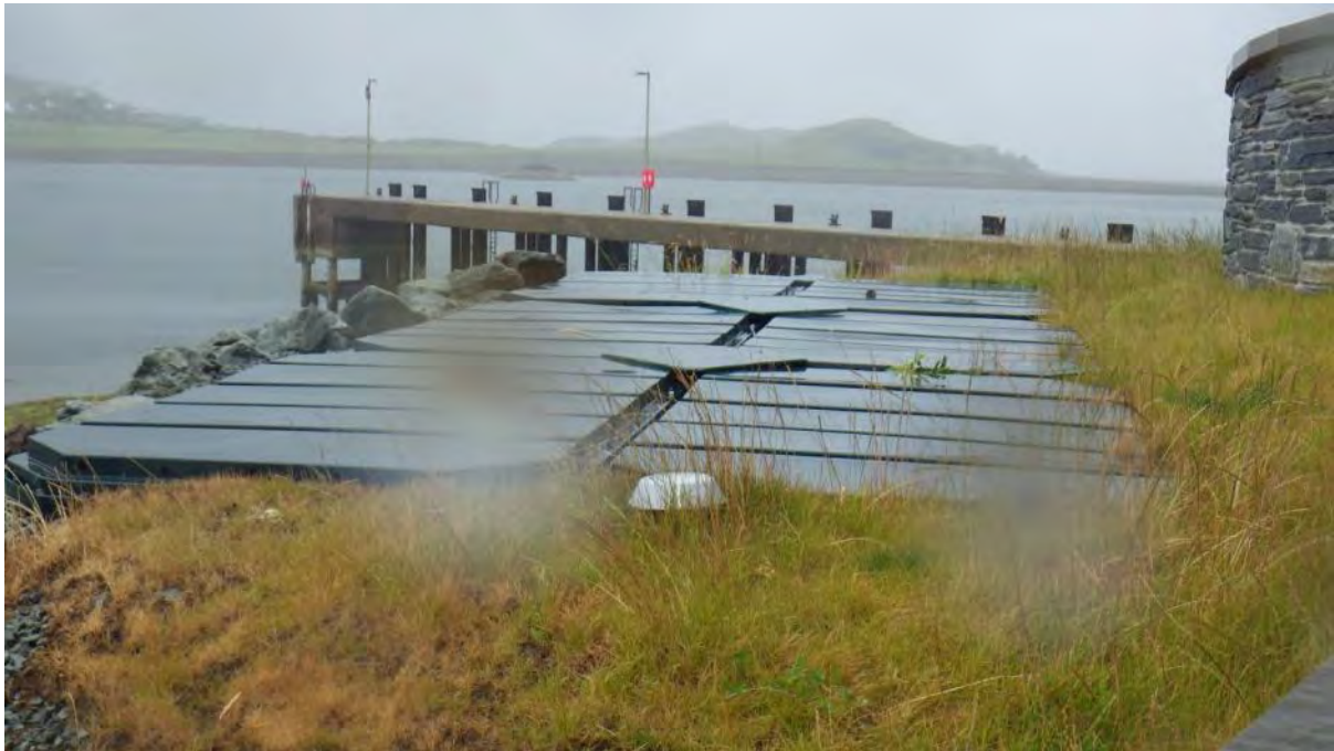
Figure 9. Septic tank over the wall from car park at Sconser Pier. Associated with WP20.
