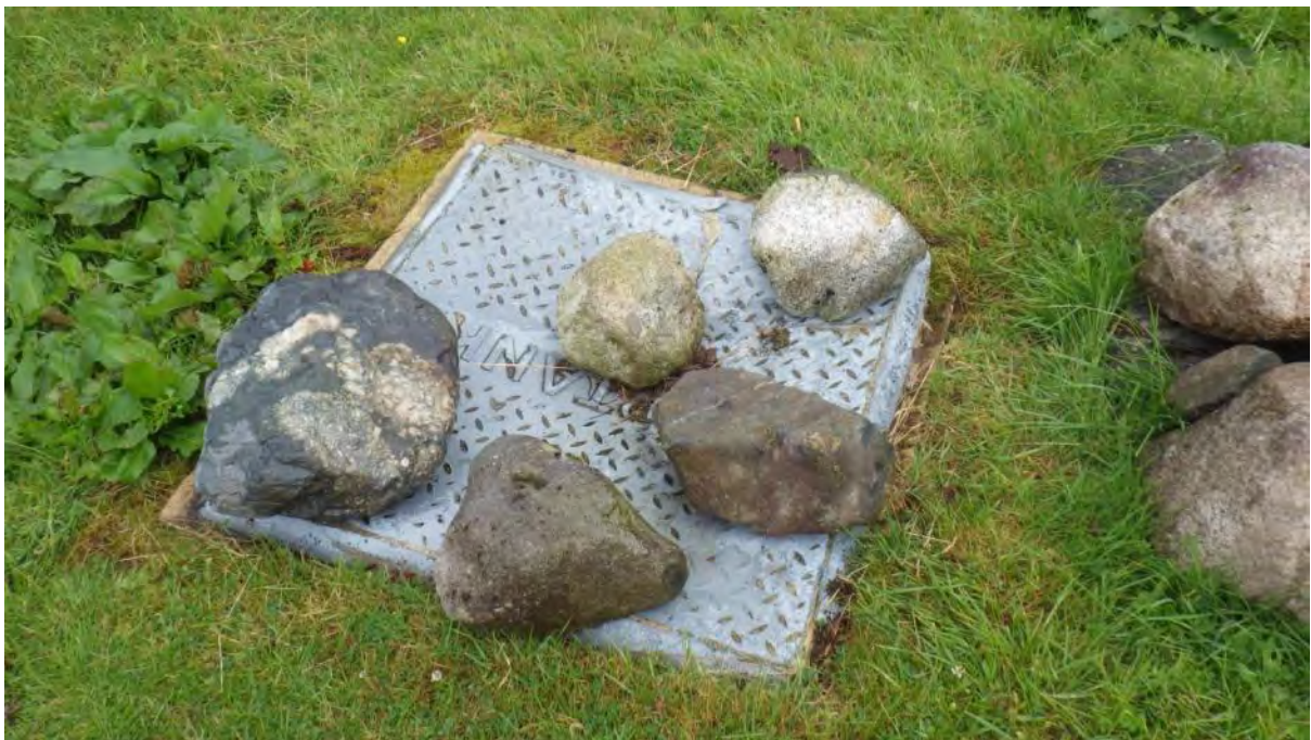
Figure 8. Septic tank on campsite grounds. Associated with WP10.
