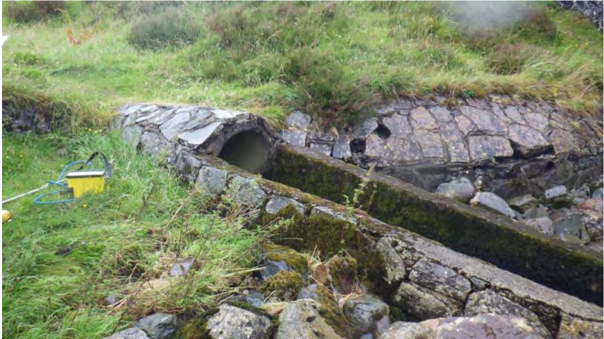
Figure 7. Discharge pipe running under A863 road into river. Site of LSFW1. Associated with Waypoint (WP) 3.
