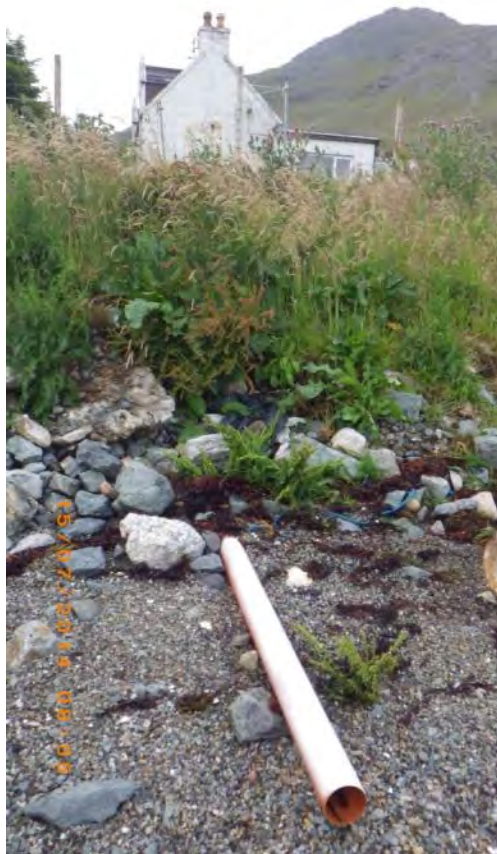
Figure 12. Discharge to seawater, pipe below house protruding onto shore. Site of LSSW2. Associated with WP 29.
