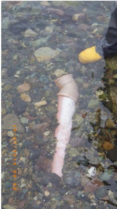
Figure 13. Submerged discharge pipe. Site of LSSW3. Associated with WP39.
