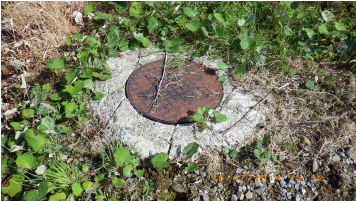
Figure 17. Possible soakaway. Associated with WP70.
