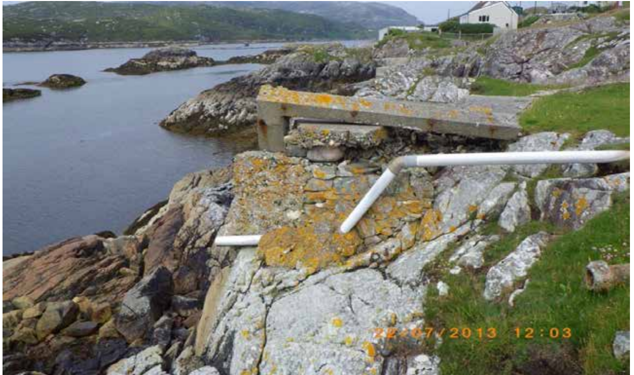
Figure 10. Pipe coming from septic tank no outflow. Waypoint 11.
