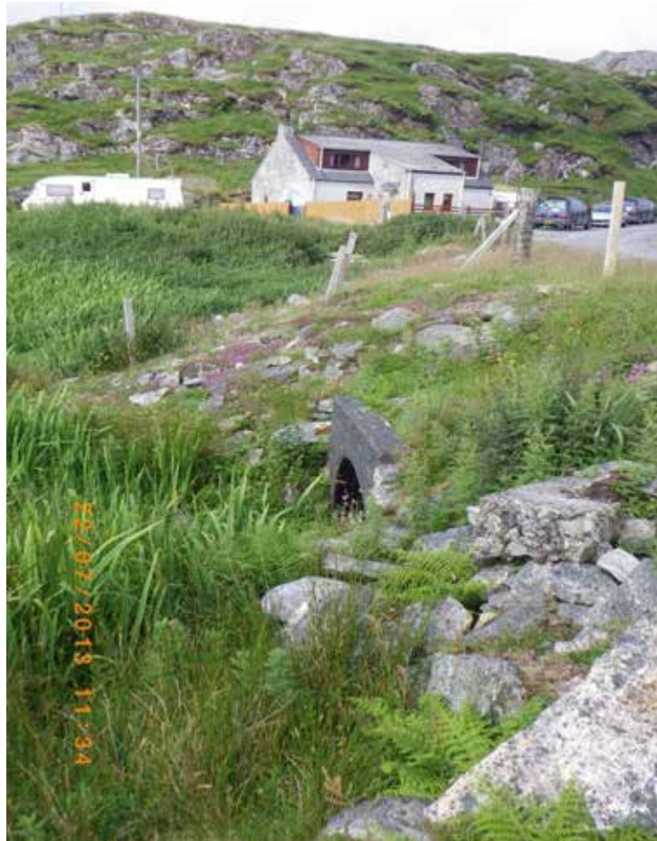
Figure 5. Tunnel directing watercourse from under road. Waypoint 6. Location of sample LSTFW1.
