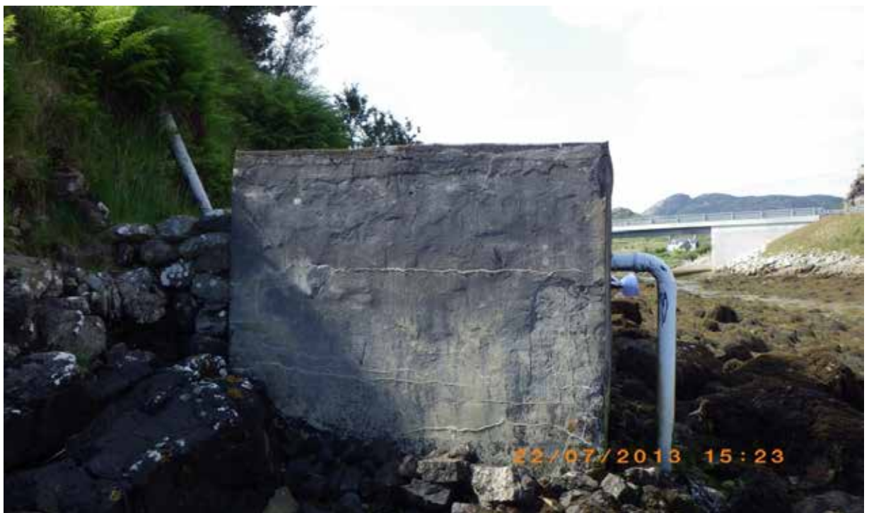
Figure 15. Septic tank from private dwelling. Waypoint 32.
