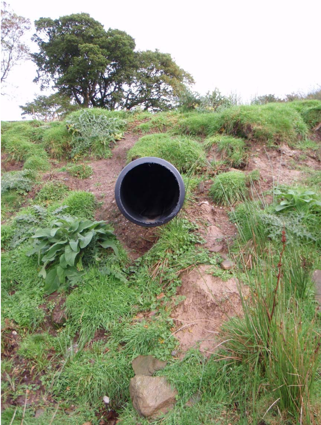
Figure 30. Dry pipe, evidence of previous flow
