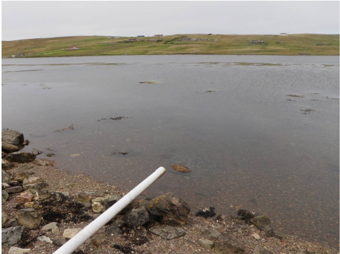
Figure 18 Active discharge pipe, Seli Voe south shore
