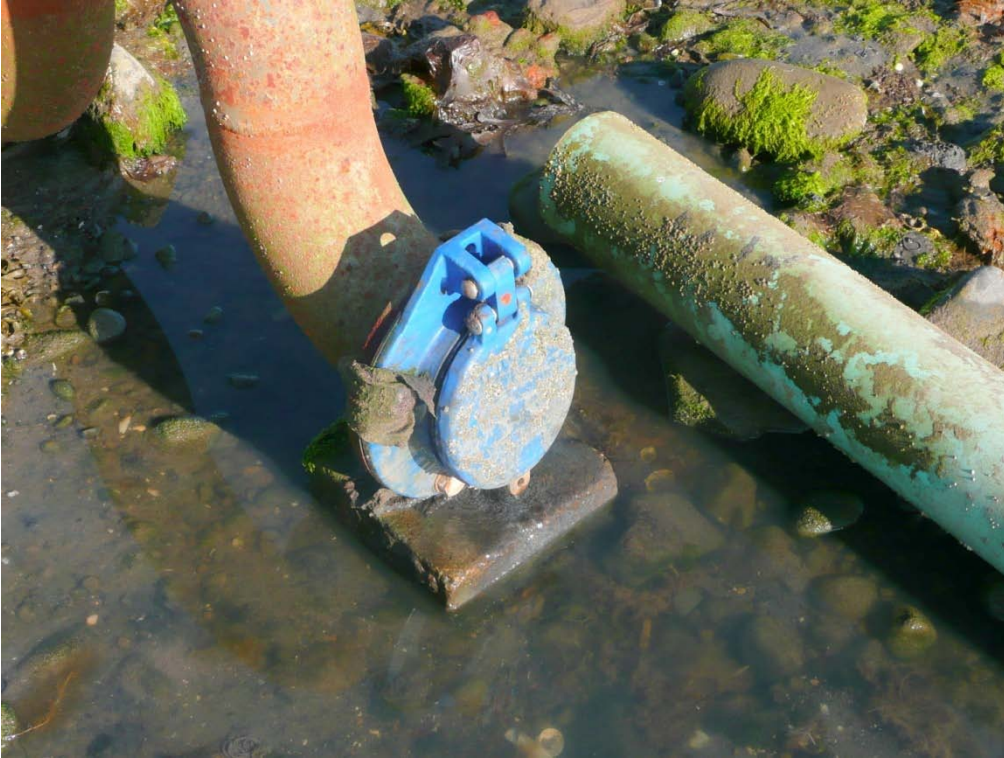
Figure 16. End of outfall pipe shown in figures 15 & 16, location of sea water sample LB008
