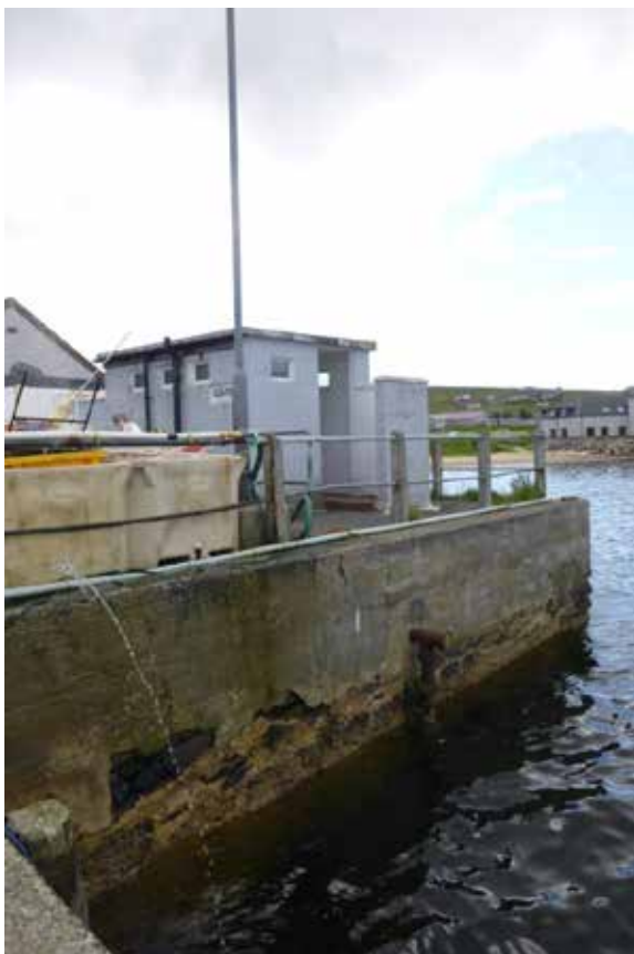
Figure 9 – Public toilets at the Linkshouse Pier, pipe leading to the sea possibly associated with discharge from the toilets.
