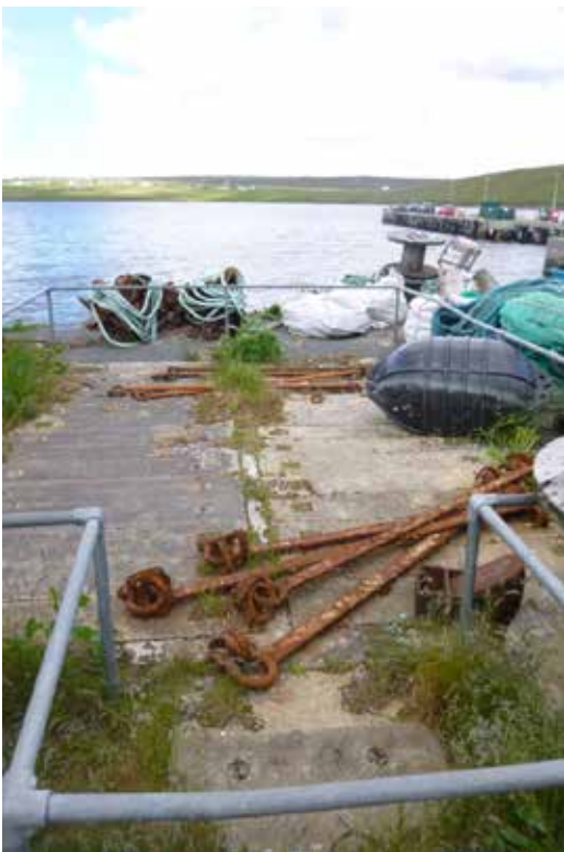
Figure 11 – Linkshouse Septic Tank adjacent to the Linkshouse Pier.
