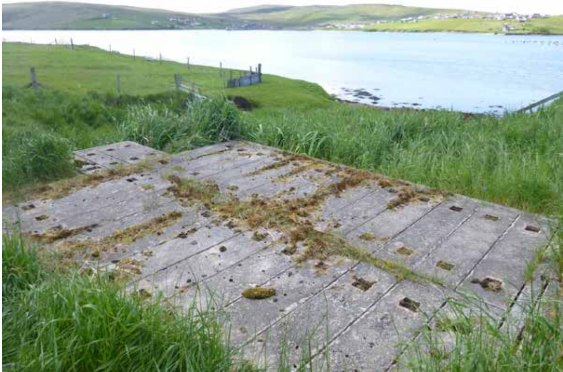
Figure 6 – North a Voe Septic Tank
