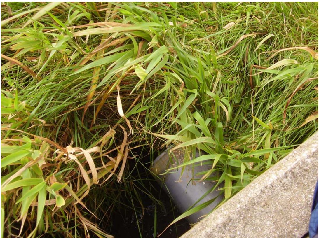
Figure 27. Discharge from tank drains into this hole
