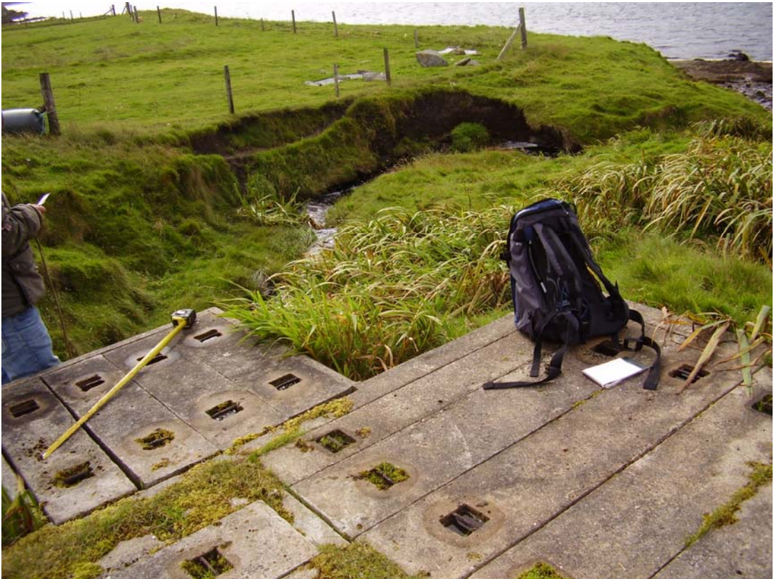
Figure 26. Septic tank cover
