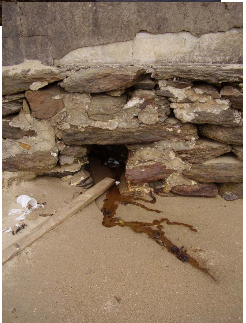
Figure 7. Seepage on shore
