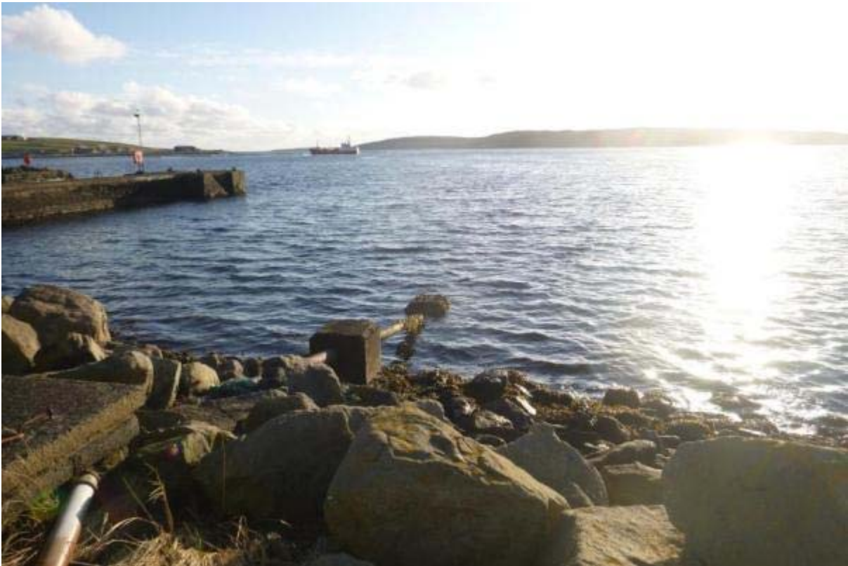
Figure 16 – Outflow from septic tank below public toilets.
