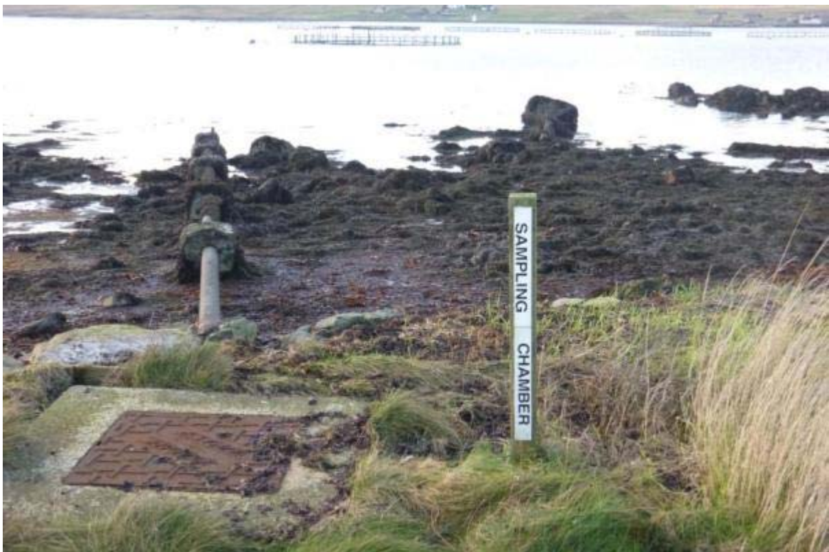
Figure 7 – Outfall pipe for Uyeasound STW Community discharge.
