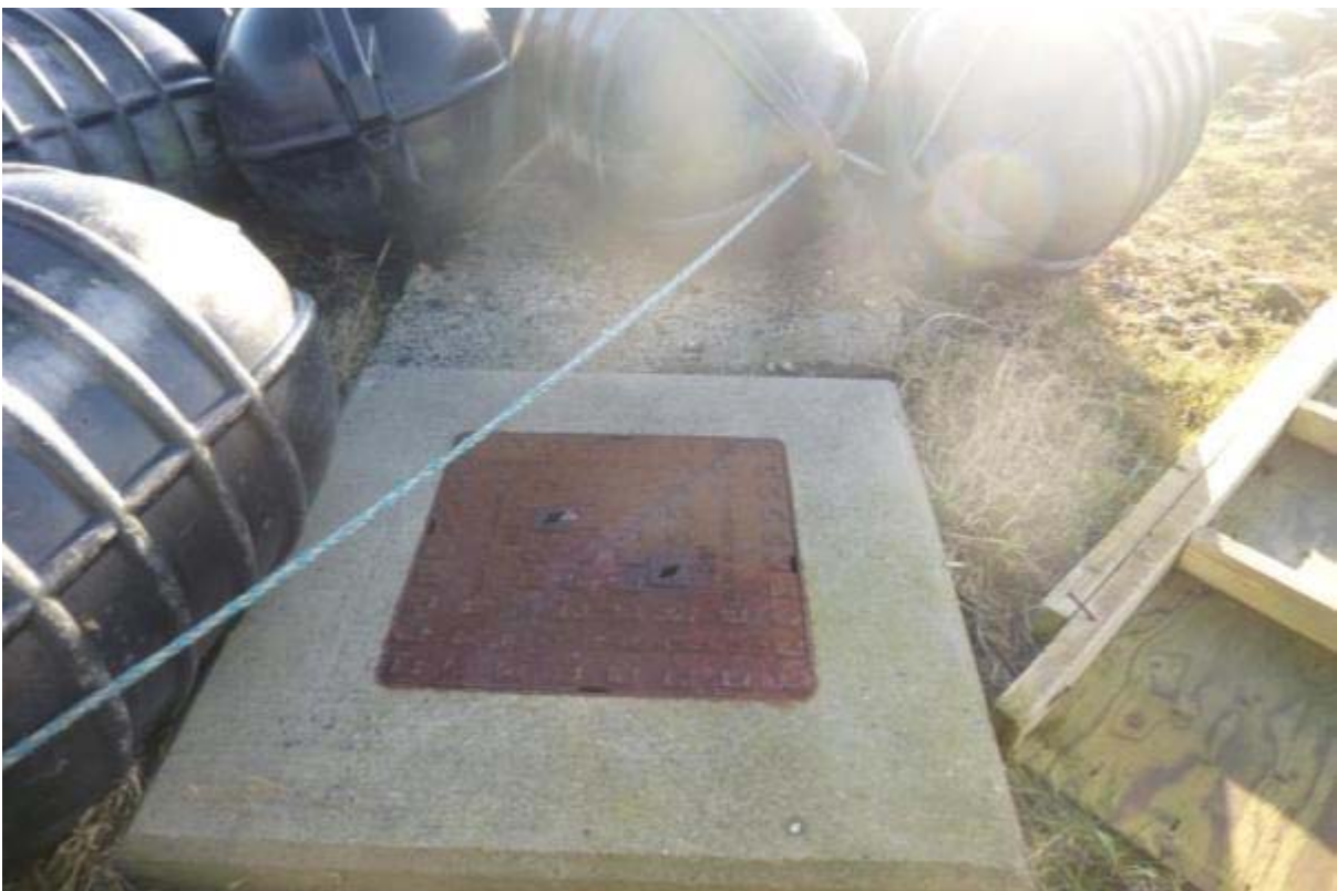
Figure 15 – Septic tank associated with public toilets.
