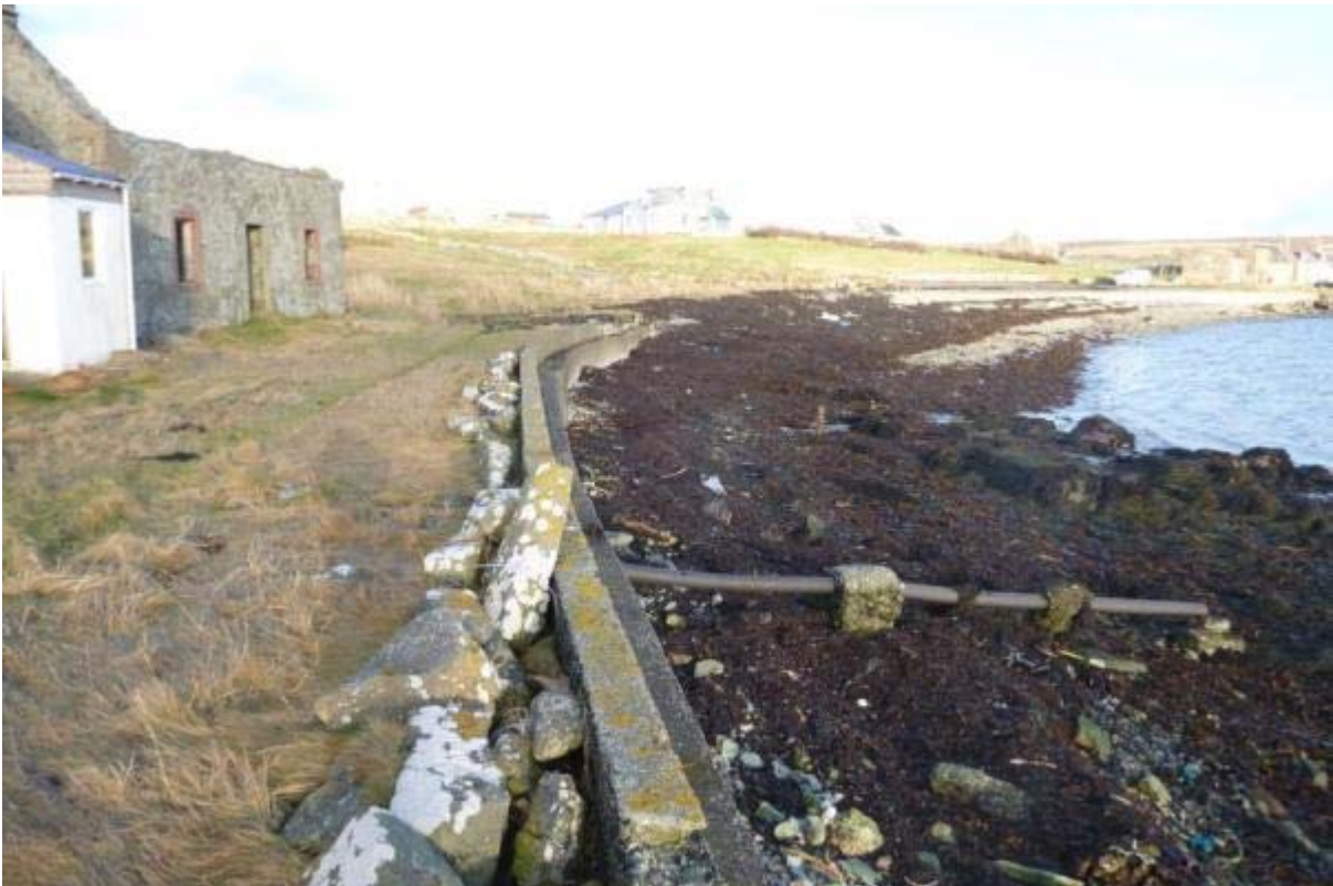
Figure 17 – Plastic pipe with no outflow on western shoreline.
