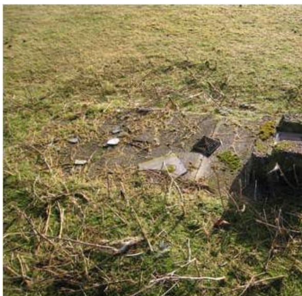
Figure 56. Septic tank at NF 00220 92590
