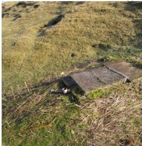
Figure 55: Septic tank at NF 00070 92530
