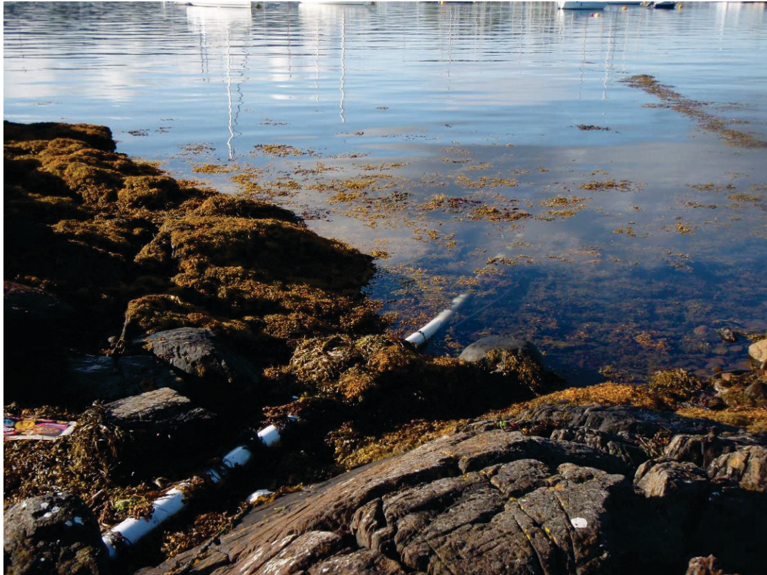
Figure 9. Septic tank outfall pipe from house/holiday home
