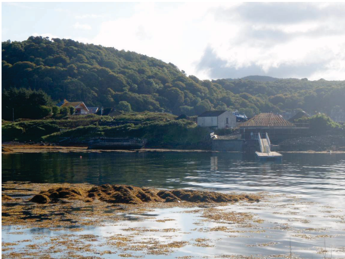
Figure 10. Construction of one new house and demolition of old house on Rubh'a Chruidh Island
