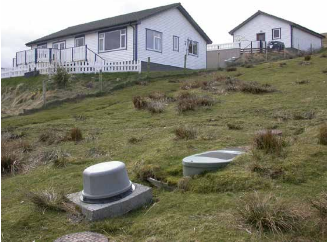
Figure 10 – Septic tank of an occupied property at Hoga, west of Voe.
