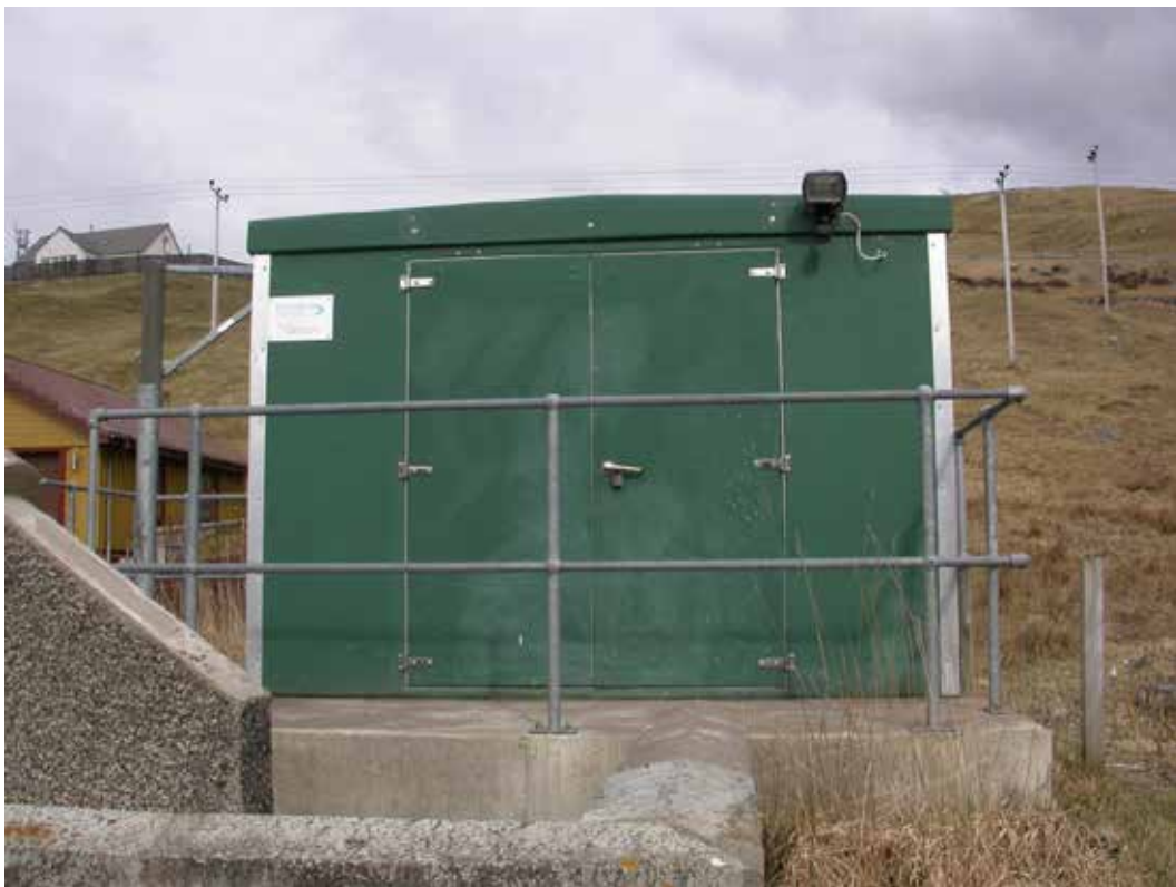
Figure 11 – Voe pumping station.
