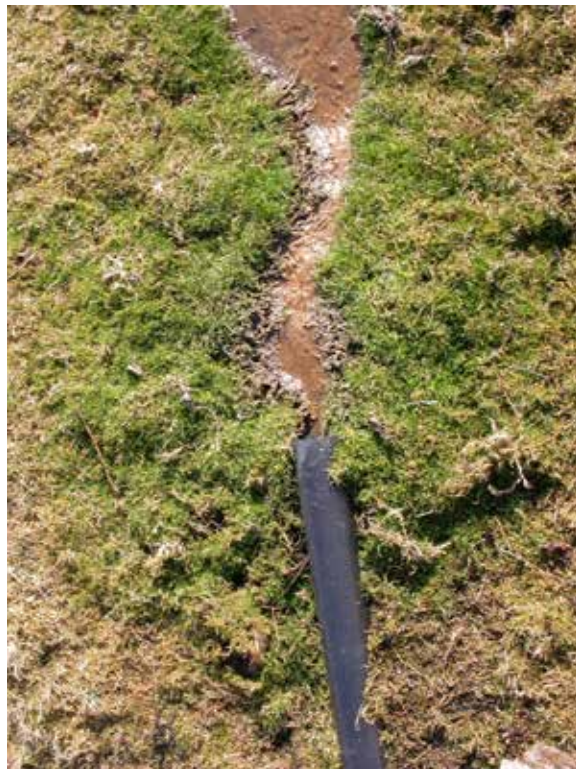
Figure 13 – Overflow pipe of a septic tank discharging to the shore associated with a property east of the Pinchdyke fishery.
