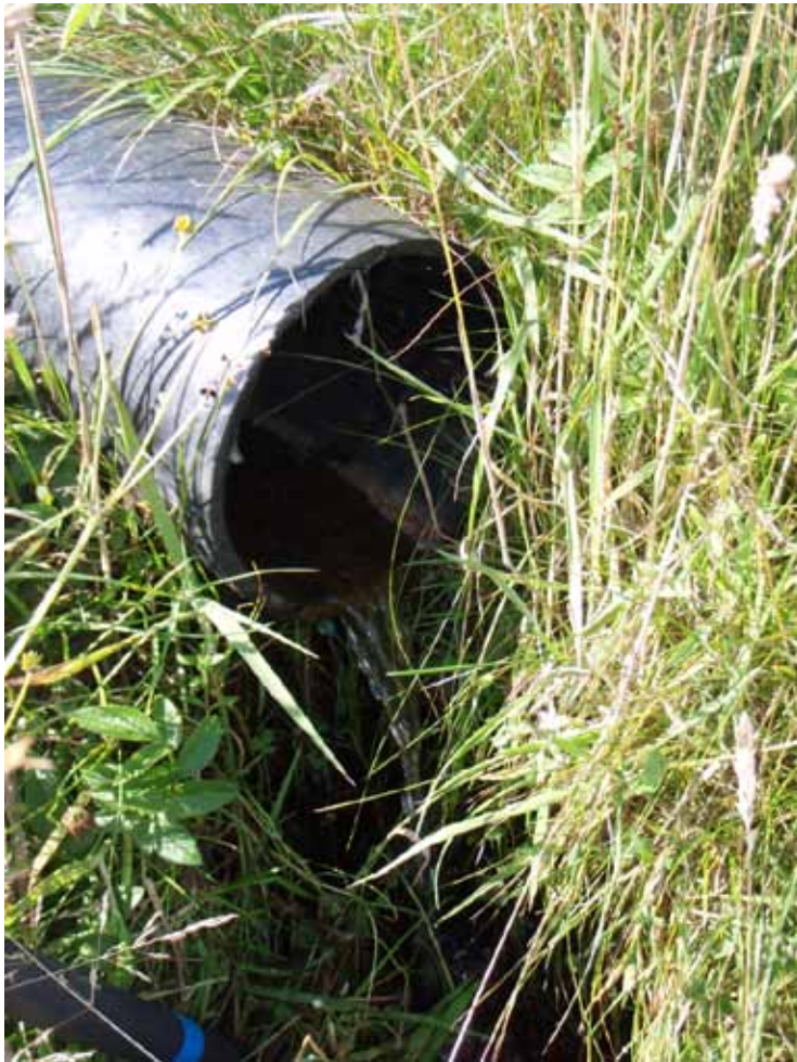
Figure 15. Flowing outfall pipe, location of freshwater sample MRFW5
