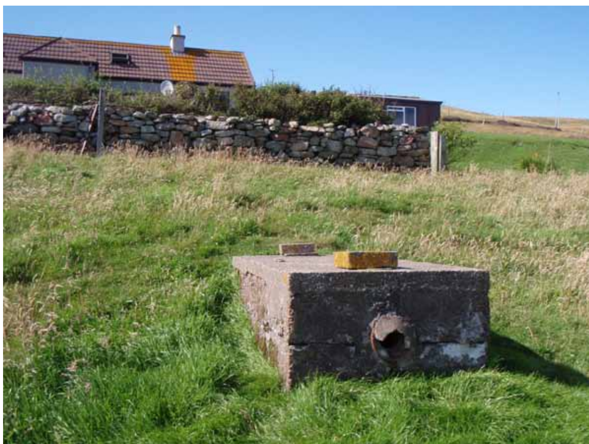
Figure 11. Outfall pipe and septic tank leading down from house, no flow
