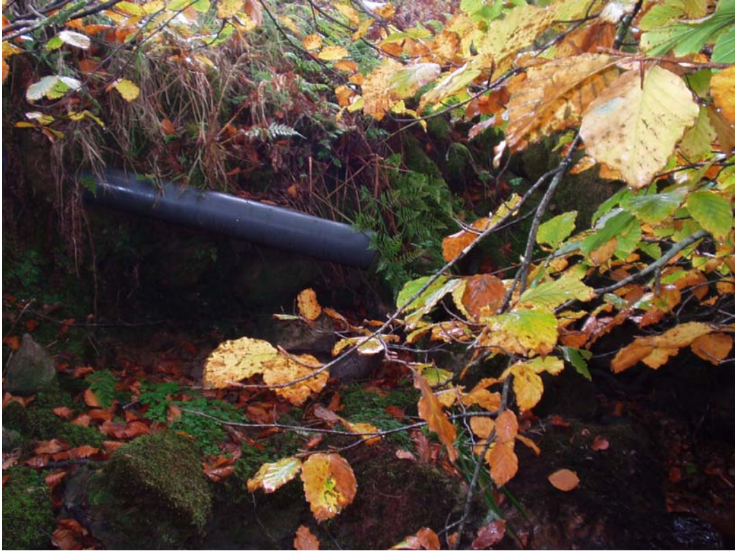
Figure 8. Grey pipe going into stream at Bunlarie
