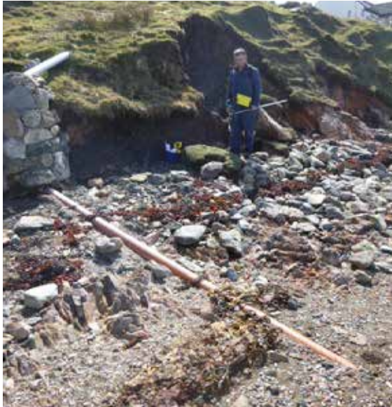
Figure 6 – Bed and Breakfast property pipe from the septic tank entering the water south of the Sandsound Voe fishery.
