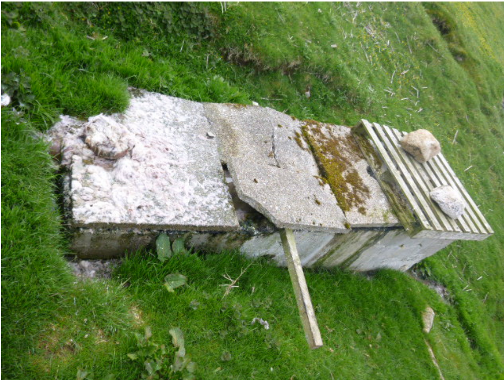
Figure 5 – Overflowing septic tank at the south end of Sandsound Voe.
