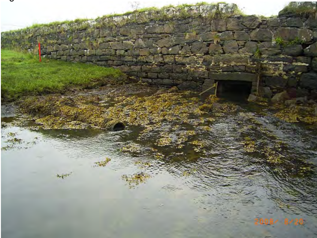
Figure 12 Sewer outflow to stream at Balvicar
