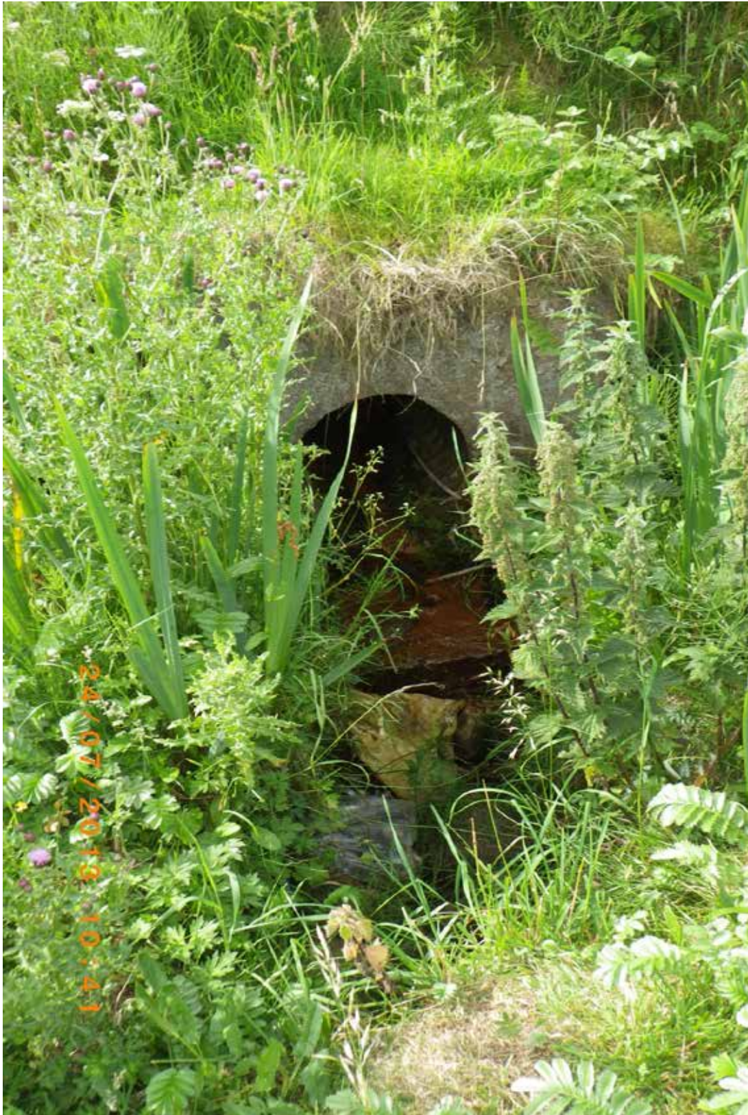
Figure 9. Watercourse piped under road onto shore from hill. Associated with waypoints 24 and 25. Planned freshwater sample LSFW8
