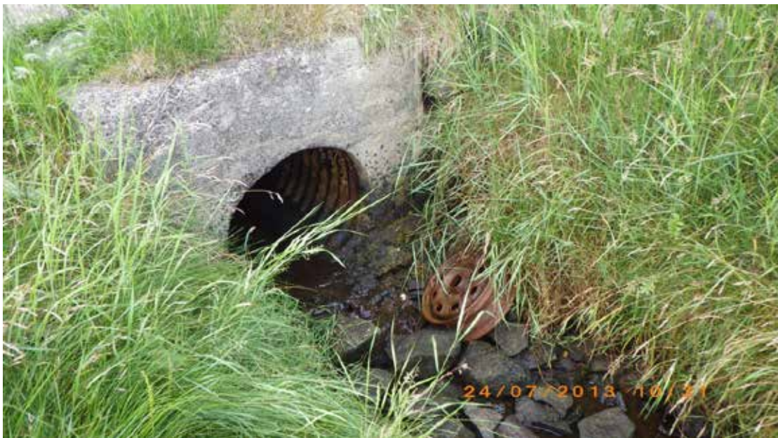
Figure 8. Concrete pipe directing a burn under the road from a hill onto shore. Associated with waypoints 22 and 23. Planned freshwater sample LSF7.
