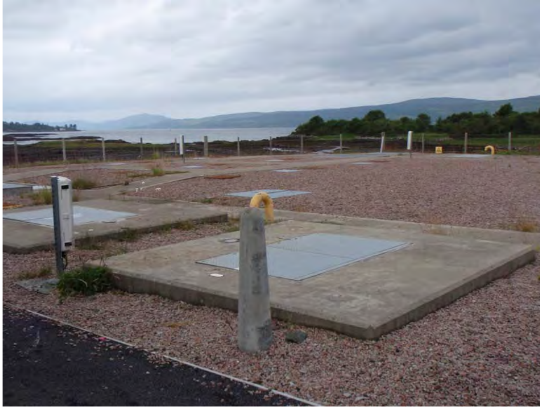
Figure 21. Corner of Salen Treatment works
