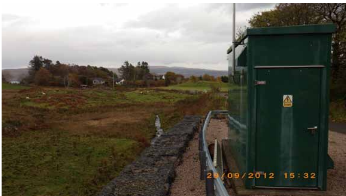
Figure 4. Pumping station beside burn next to road.
