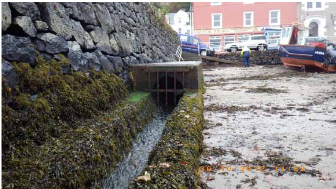
Figure 10. Smell of sewage from this stream, location of sample TOW5.
