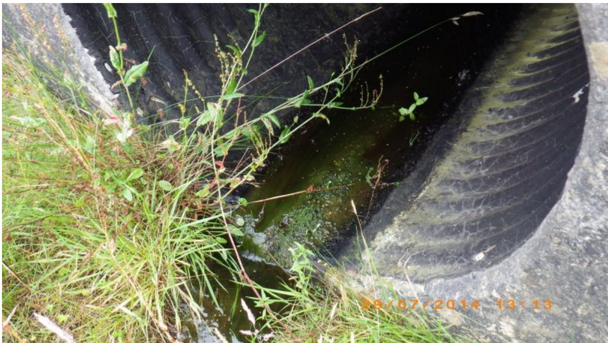
Fig. 15 Drain under roadway with almost no flow. Site of unplanned freshwater sample SFFW8, waypoint 56.
