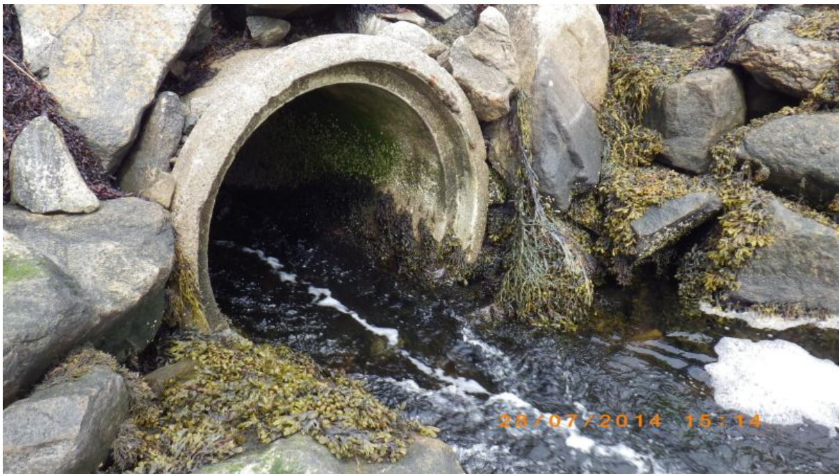
Fig. 9 Tidal freshwater outlet drain under roadway sampled at low tide. Site of planned freshwater sample SFFW3. Waypoint 25.
