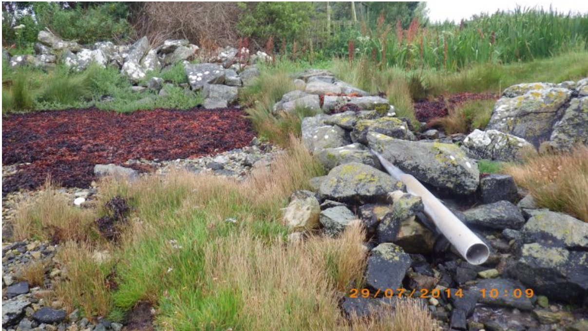
Figure 10. Septic tank discharge onto the shore, south east of the causeway. Site of unplanned freshwater (contaminated) sample SSFW4. Waypoint 35.
