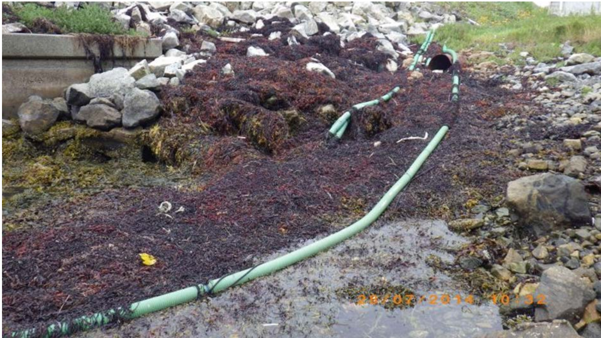
Fig. 8 Seawater intake and outfall pipes at “Sutherland Game and Shellfish” plant. Waypoint 12.
