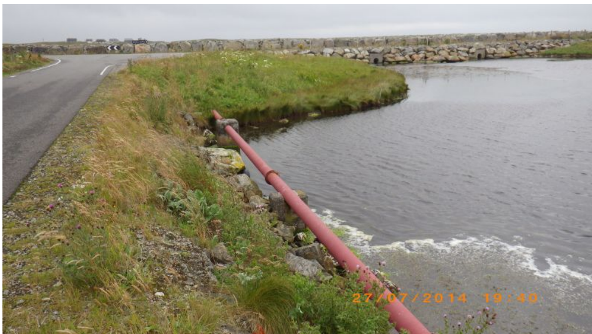
Figure 5. Lochdar septic tank pipe falling towards the shoreline, situated southwest of the survey site. Waypoint 5.
