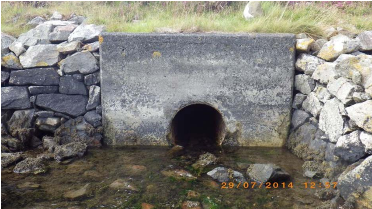
Fig. 14 Drain under roadway with slow flowing watercourse. Site of unplanned freshwater sample SFFW7, waypoint 54.
