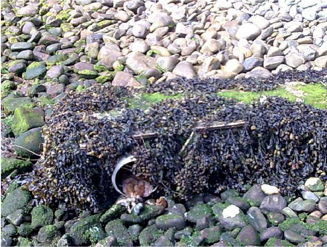
Figure 24. Outfall with solid waste evident, waypoint 99.
