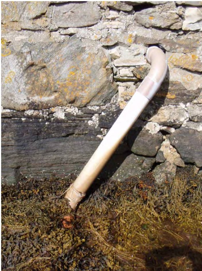
Figure 11. Discharge pipe behind toilet block.
