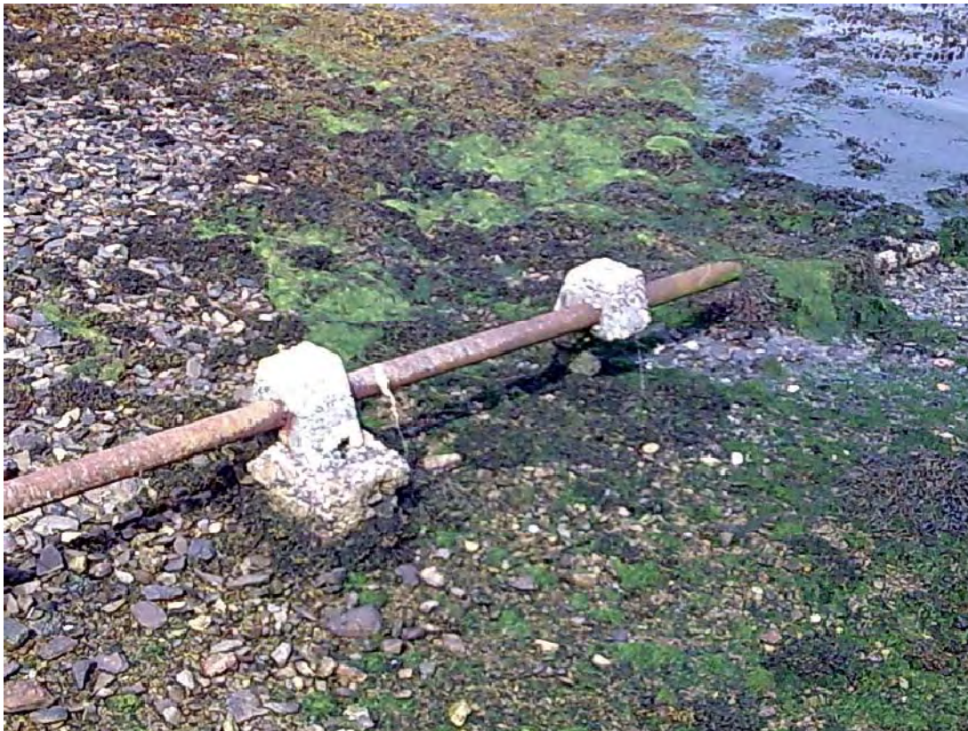
Figure 27. Discharge pipe adjacent pier, dribbling from end.
