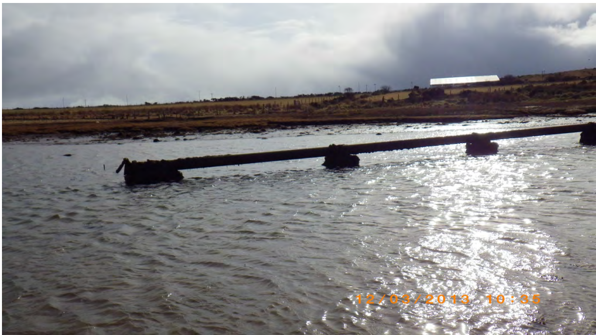
Figure 12. Waypoint 29 & 30. Large cast iron discharge pipe with storm valve on end. Site of sample TSW9.
