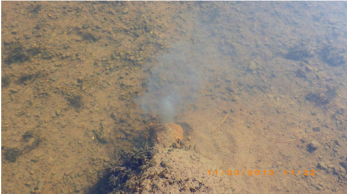
Figure 7. Waypoint 15 & 16. Cast iron discharge pipe encased in concrete. Looks contaminated. Site of sample TSW4.
