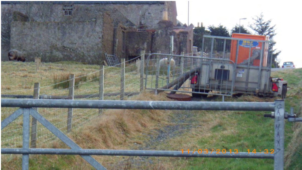
Figure 10. Waypoint 24 & 25. Land drainage and open man-hole cover with pump. Site of sample TSW8.
