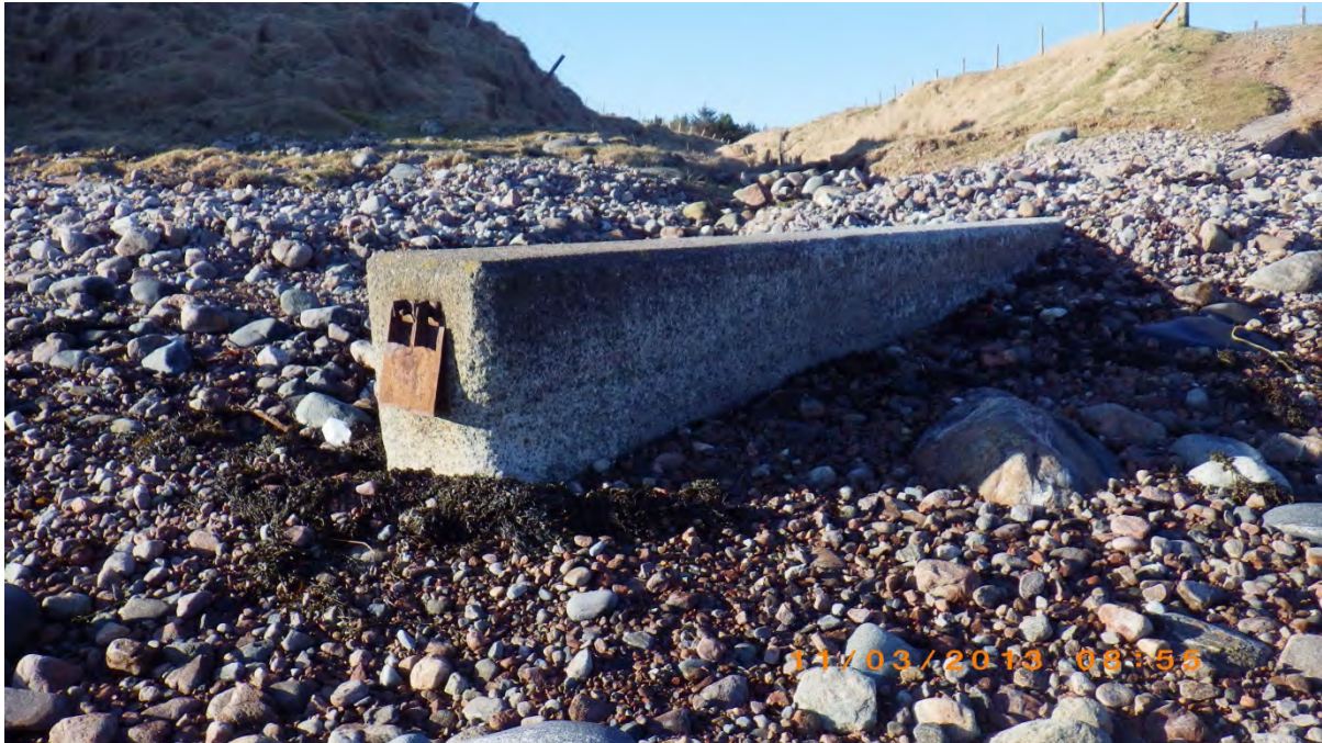
Figure 3. Waypoint 1. Discharge pipe encased in concrete, no discharge visible.
