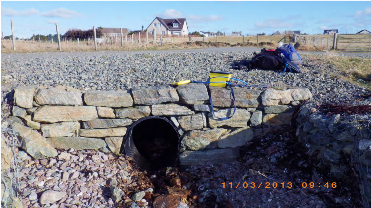
Figure 5. Waypoint 5 & 6. Pipe running under road onto the shore with discharge coming from pipe. Site of sample TSW1.
