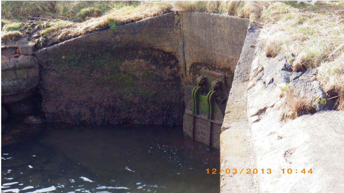
Figure 13. Waypoint 31 & 32. Storm culvert draining land area behind. Site of sample TSW10.
