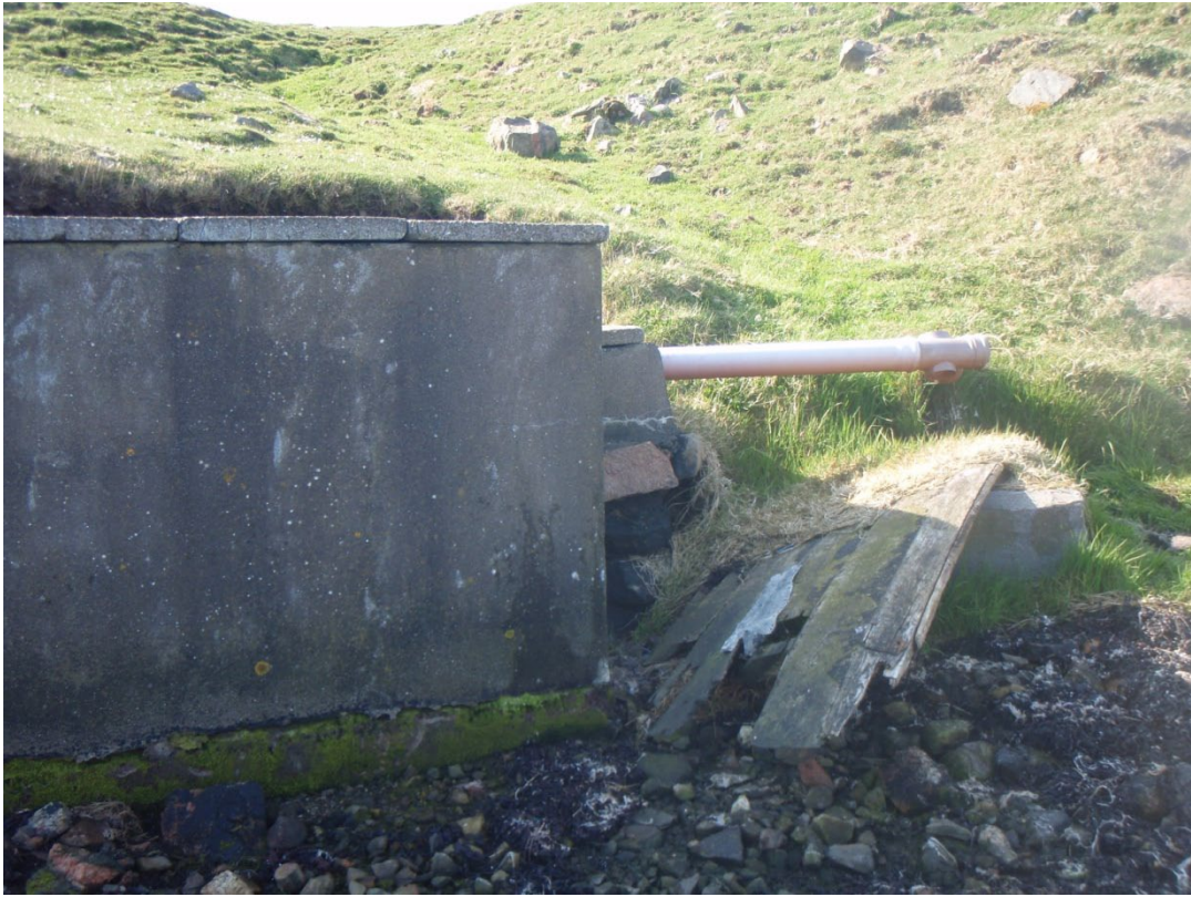
Figure 4. Septic tank and outfall pipe
