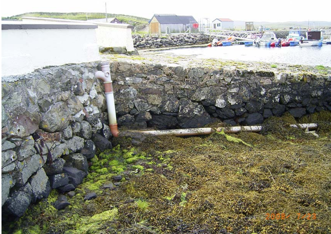
Figure 21 Private septic outfall
