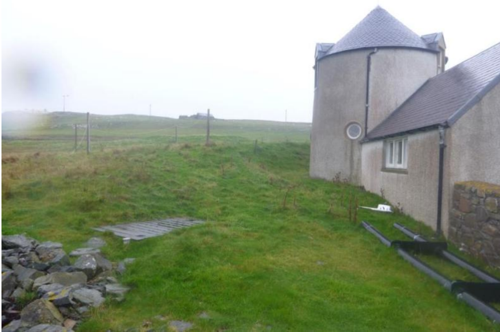
Figure 12 – A concrete septic tank with outflow to Lera Voe.
