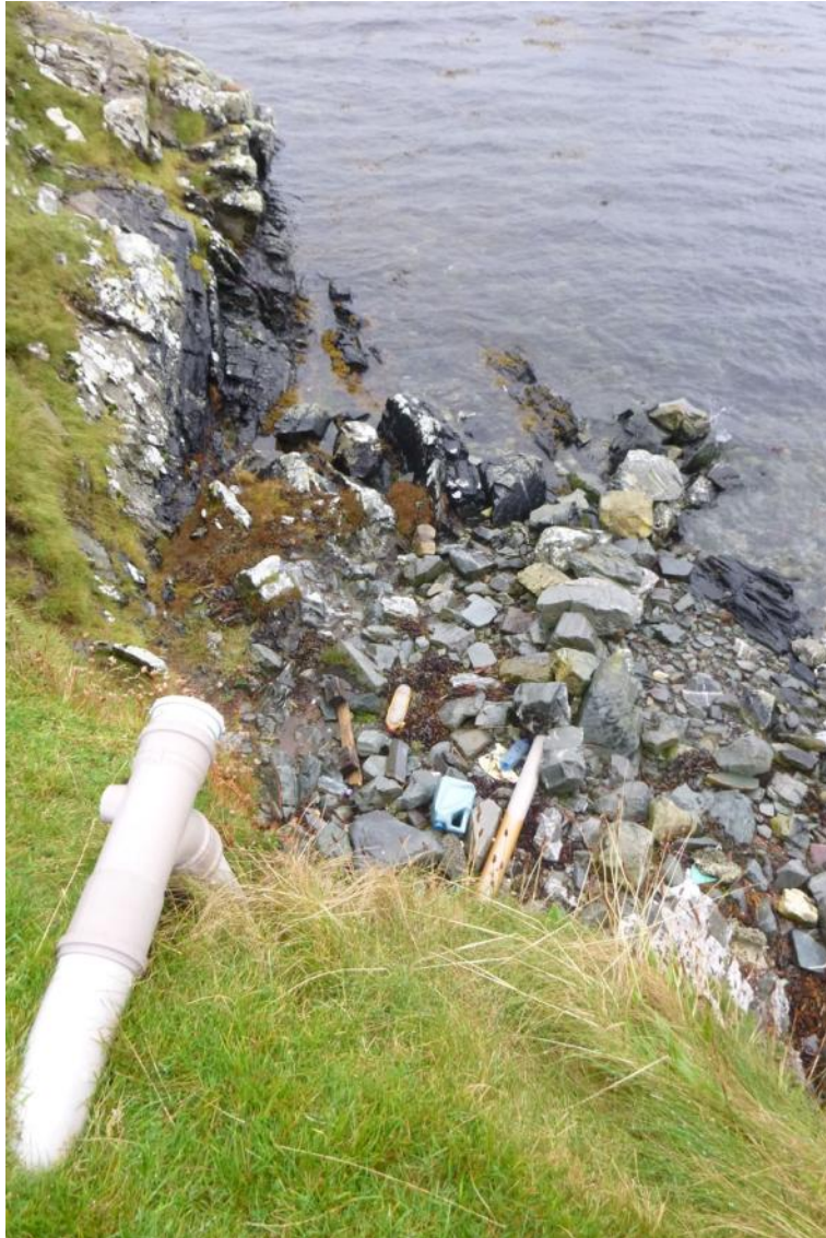
Figure 15 – A plastic pipe leading into the sea at Riskaness
