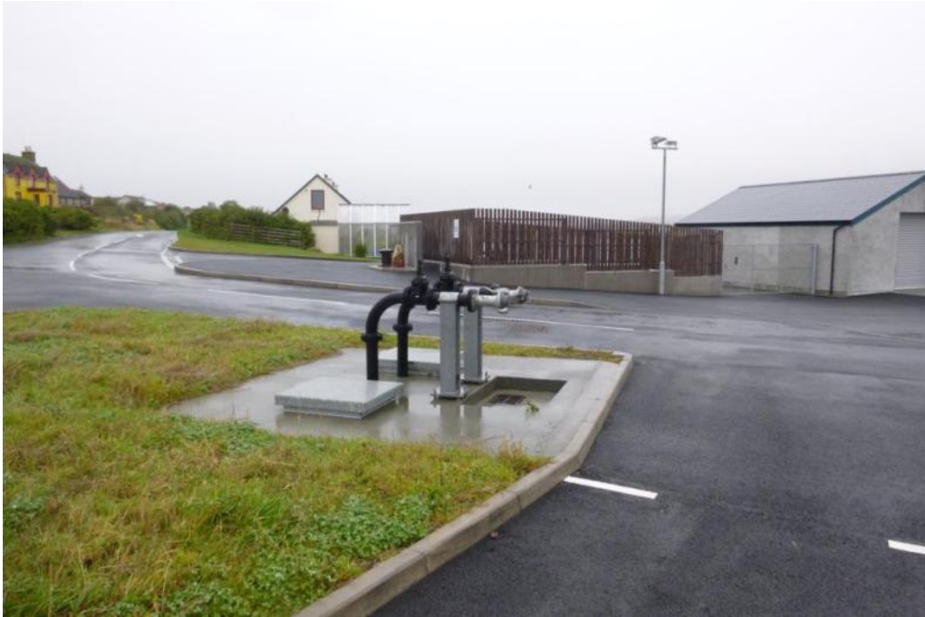
Figure 20 – The Walls septic tank at head of pier.
