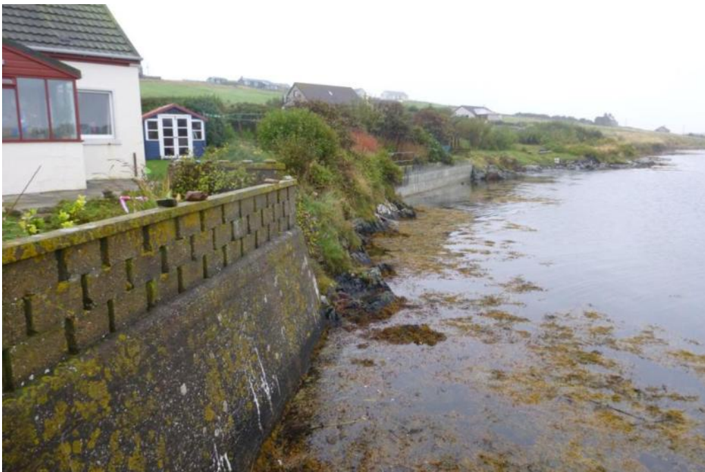
Figure 21 – A house in close proximity to shoreline at Pier Road.
