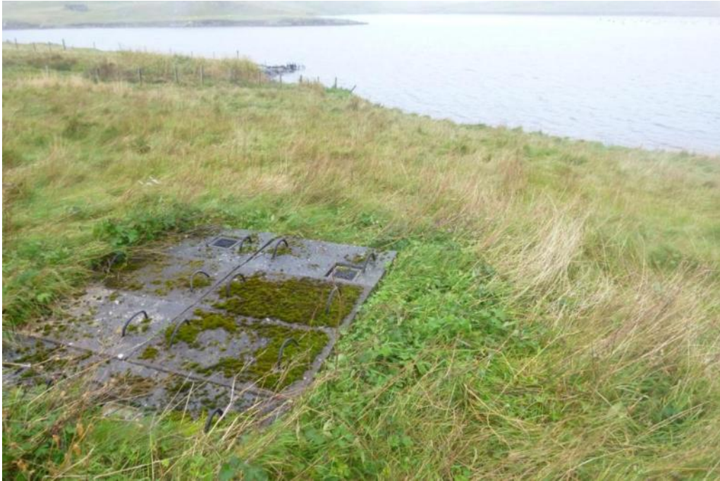
Figure 10 – A concrete septic tank on hill above the shore at Lera Voe.
