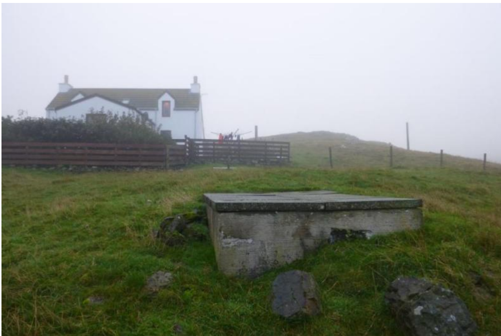
Figure 23 – A concrete septic tank with soakaway at West Banks.
