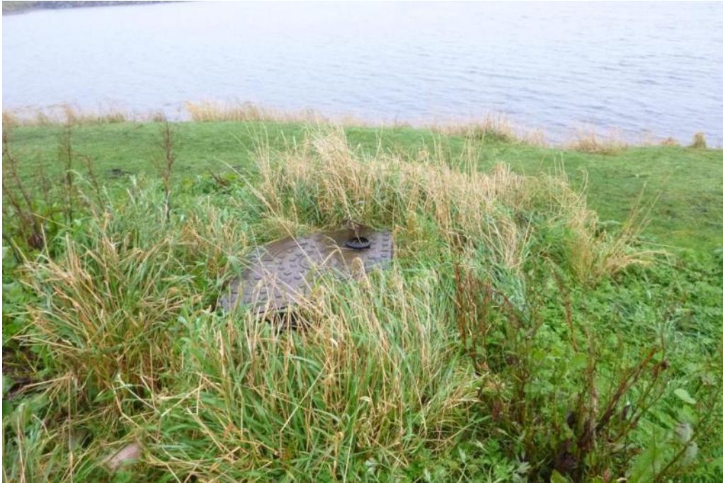
Figure 18 – A septic tank with plastic pipe disappearing underwater near Walls pier.
