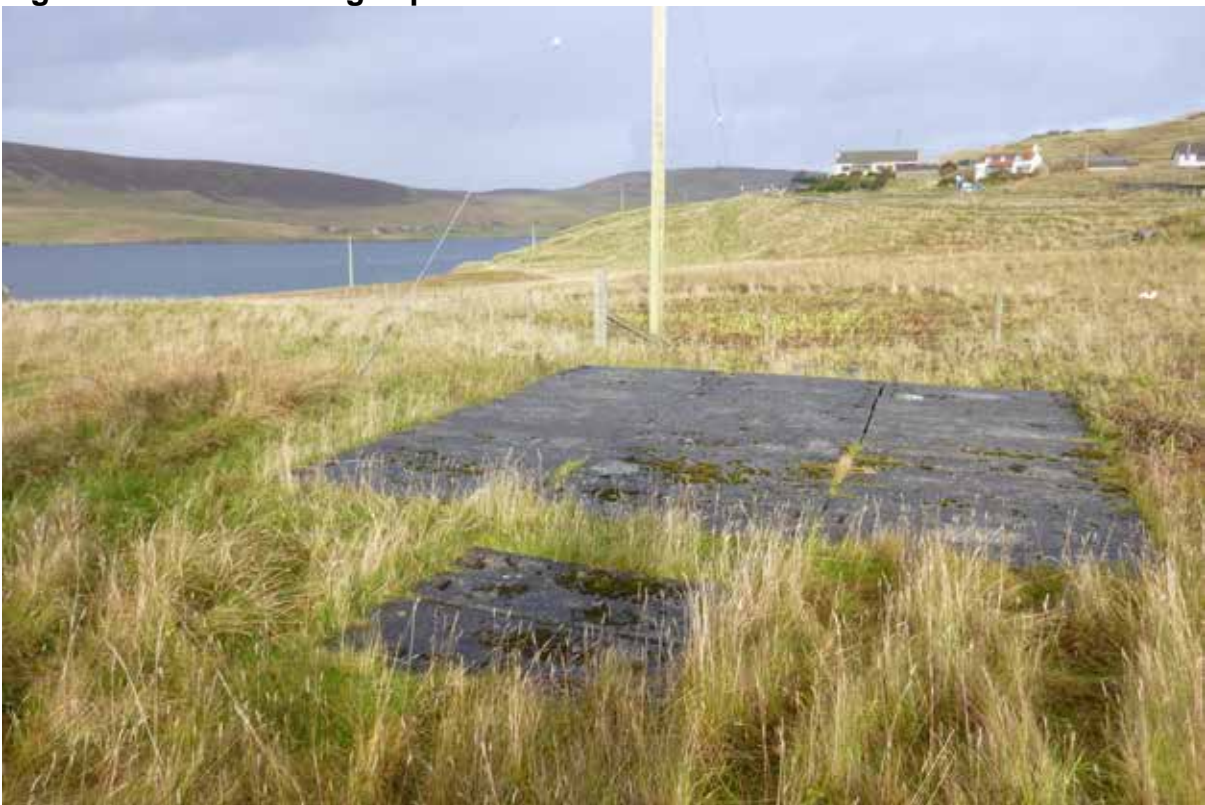
Figure 11 – Clach-na-Strom community septic tank.
