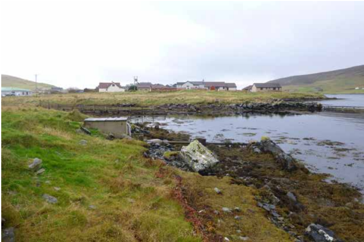
Figure 8 – Septic tank and discharge pipe at the north end of Kalliness where a seawater sample was obtained.
