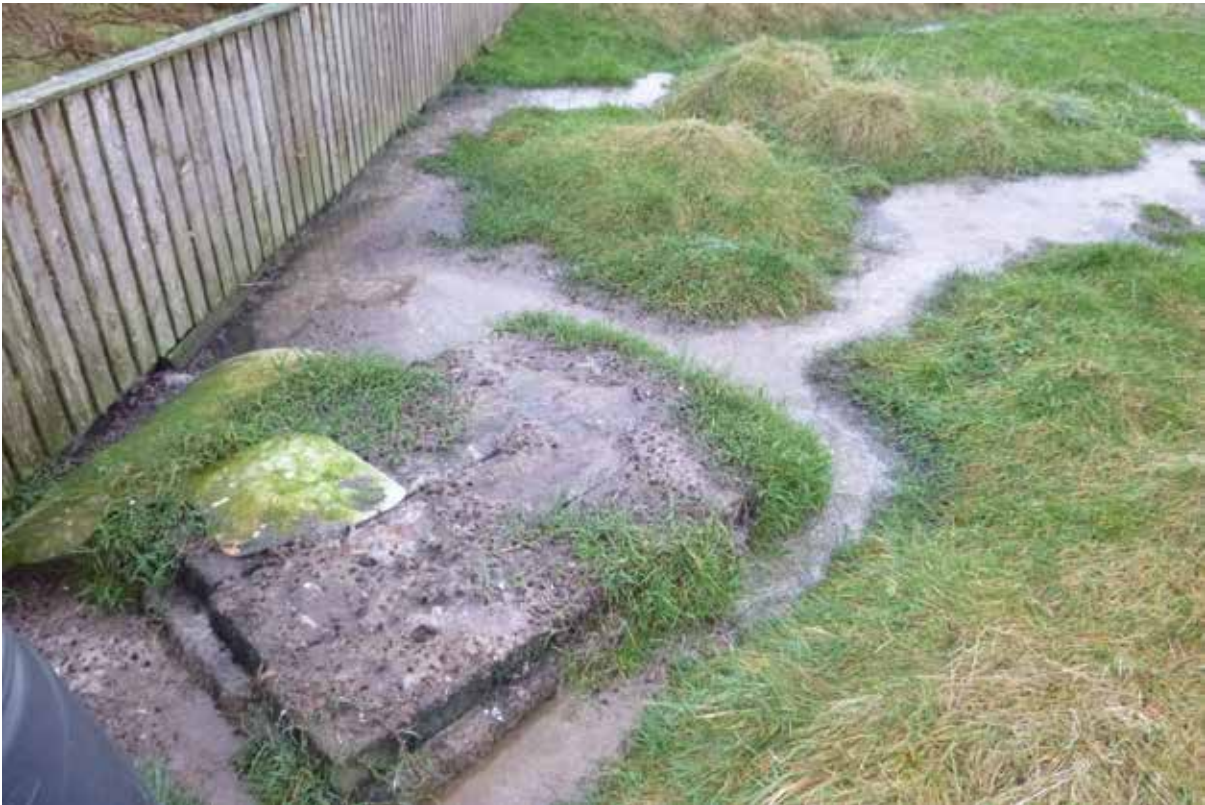
Figure 10 – Overflowing septic tank at Calder's Creek.
