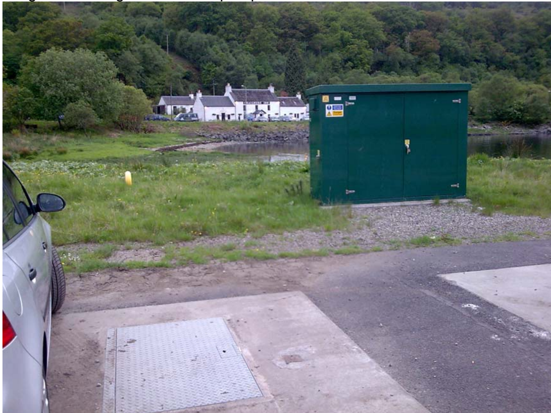
Figure 5. Criagnure WWTW pump and tanks
